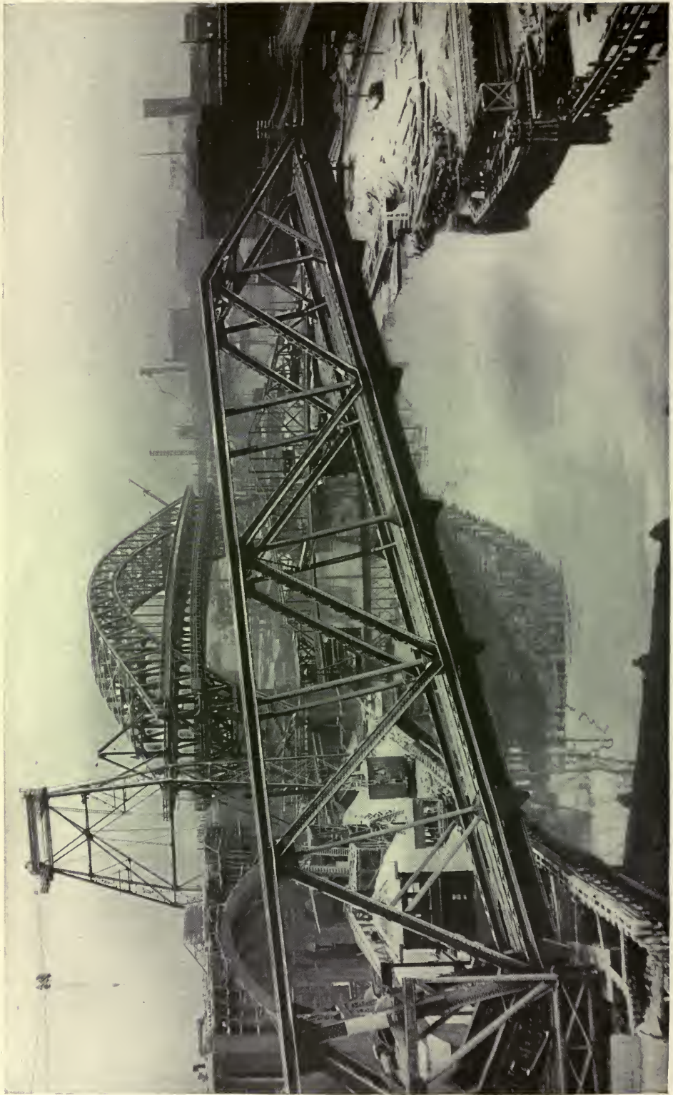
A LABYRINTH OF BRIDGES ACROSS CUYAHOGA RIVER, CLEVELAND, OHIO, INCLUDING THE NEW HIGH-LEVEL BRIDGE IN COURSE OF CONSTRUCTION
