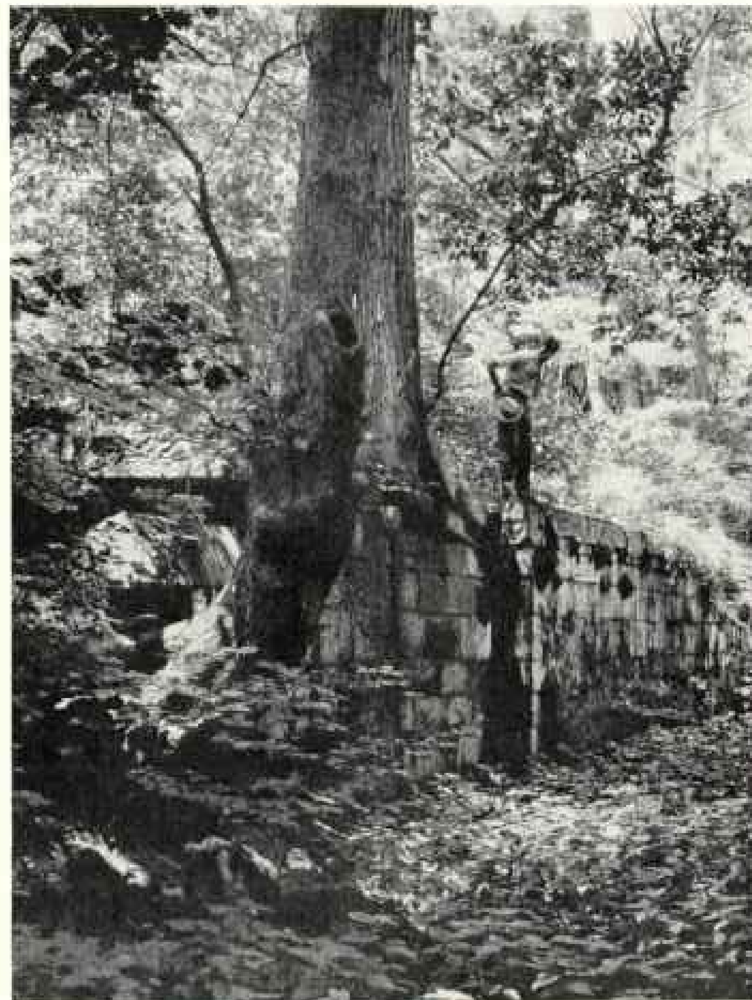
ONE OF THE SURVIVING LOCKS IN THE POTOMAC NAVIGATION COMPANY'S CANAL AT GREAT FALLS, ON THE POTOMAC
