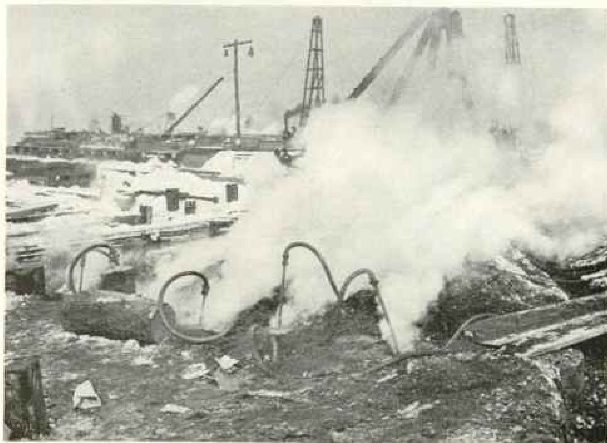
BEFORE IT WAS POSSIBLE TO PROCEED WITH EXCAVATION WORK AT HOG ISLAND LAST WINTER, IT WAS NECESSARY TO THAW THE GROUND WITH LIVE STEAM.
