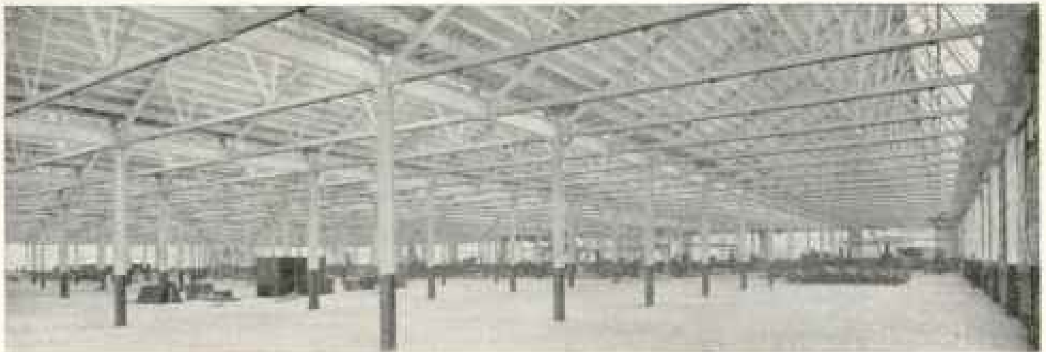
This Austin Insulated Type No. 4 Building, 300 ft. x 300 ft., a 60-day building, was ready for the Nantyk & Marmion Co., Indianapolis, two weeks ahead of time. On this performance record, the owner ordered another, and later, building.
