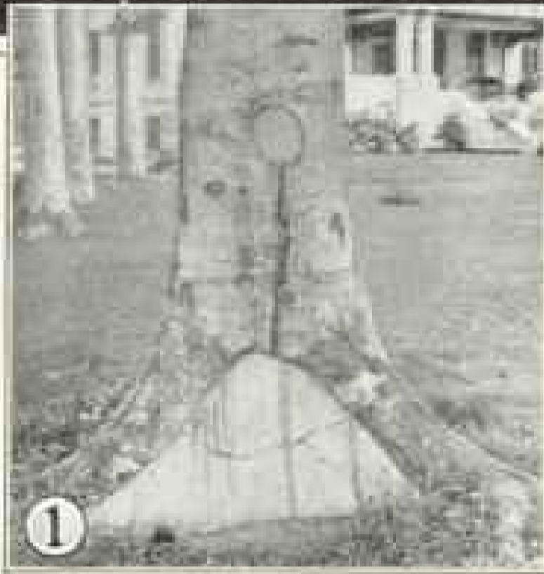
1 A crude cement patch—ineffective and injurious.
