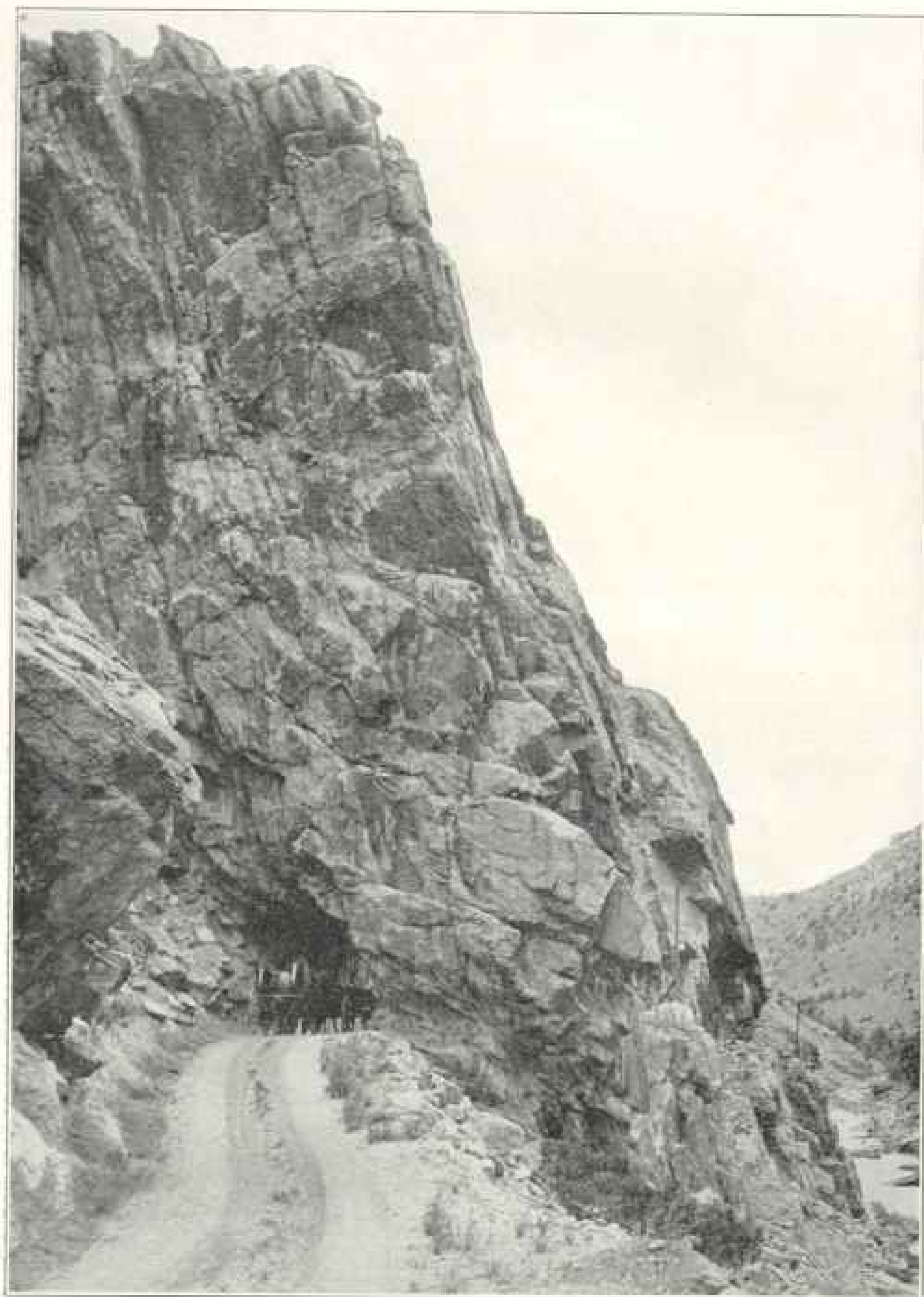
Before the engineers could begin work on the Shoshone Dam in Idaho they had to construct a road up the canyon and several times tunnel through granite mountains, as in the above picture. (See page 90)
