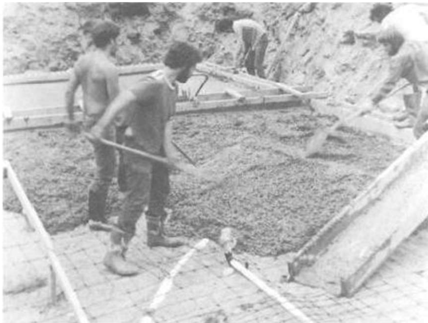
Illus. 5 11. It should be someone's job to make sure that the wire mesh is pulled up into the concrete.
