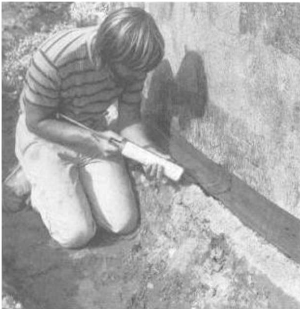
Illus. 9-1. The important detail where the footing meets the wall is sealed with a strip of Bituthene K .
