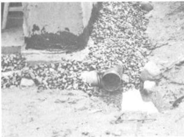
Illus. 10-4. From the southeast corner (the lowest point of the footing drain's grade) the pipe will be run at a similar slope behind the retaining wall and into a soakaway.
