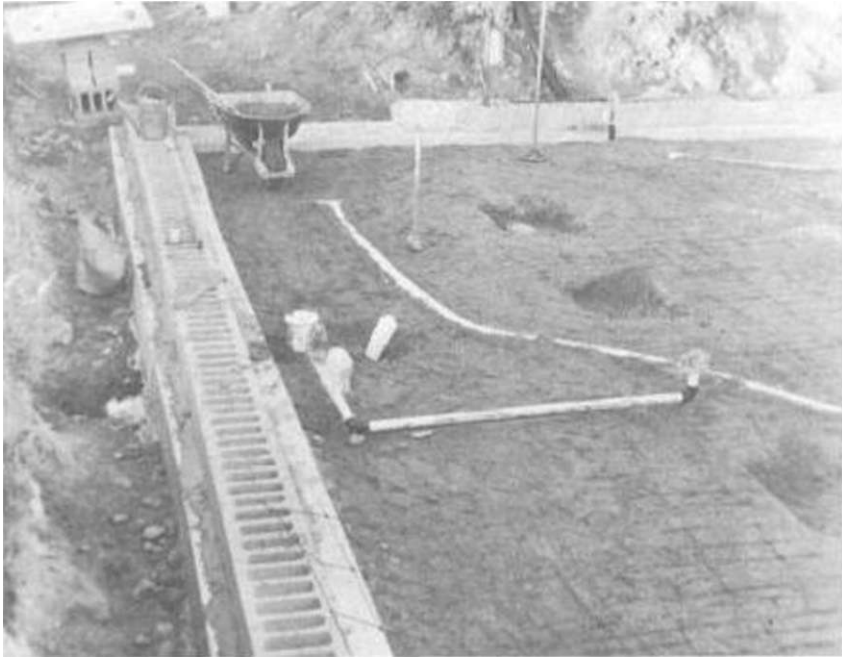
Illus. 5-8. Perforated 4" tubing was laid to remove any water that might accumulate under the floor:
