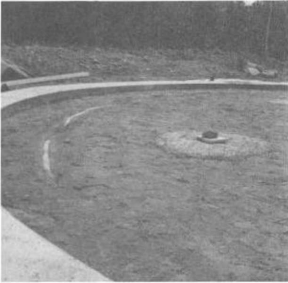
Illus. 5-6. The bottom half of the pillar footings are poured and the concrete is left rough to make a good "cold joint."
