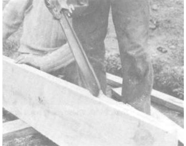
Illus. 8-9. Use a chainsaw to cut a groove down the middle of the fascia board before nailing the board into place. This groove will serve as a "drip edge" to keep rainwater from running along the underside of the roof planking and into the house.
