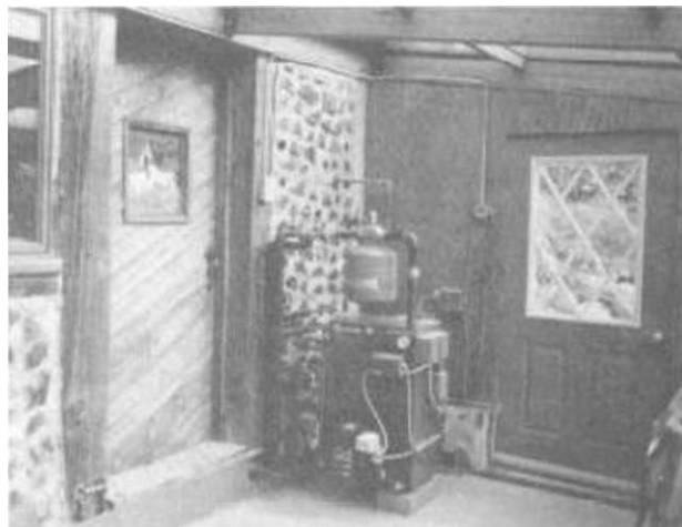
Illus. 16-5. The new oil furnace occupies a corner of the solar room.
