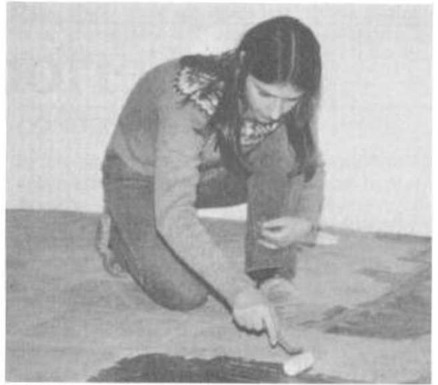
Illus. 14-7. Jaki, at Earthwood, seals the floor, which is made of roofing slates set in strong mortar.
