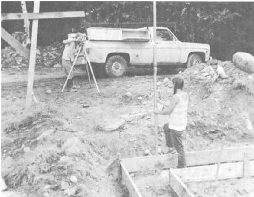
Illus. 4-9. The most important consideration when placing the footing forms is that they be level with one another.
