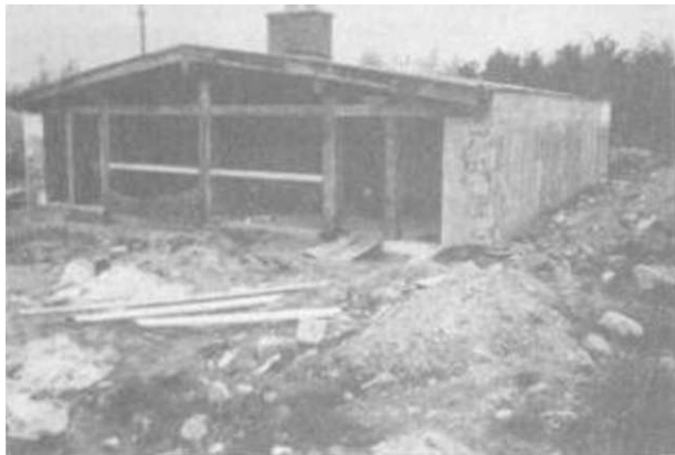
Illus. 16-4. Richard Guay's 441' x 40' Log End Cave during construction in 1980, The home is now fully earth-sheltered: berms on the north, east, and west sides: earth on the roof.
