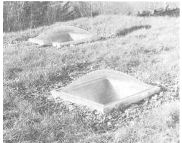
Illus. 15-1. SkvligMs, chimneys, and other roof projections should be surrounded by good drainage material, such as #2 crushed stone.
