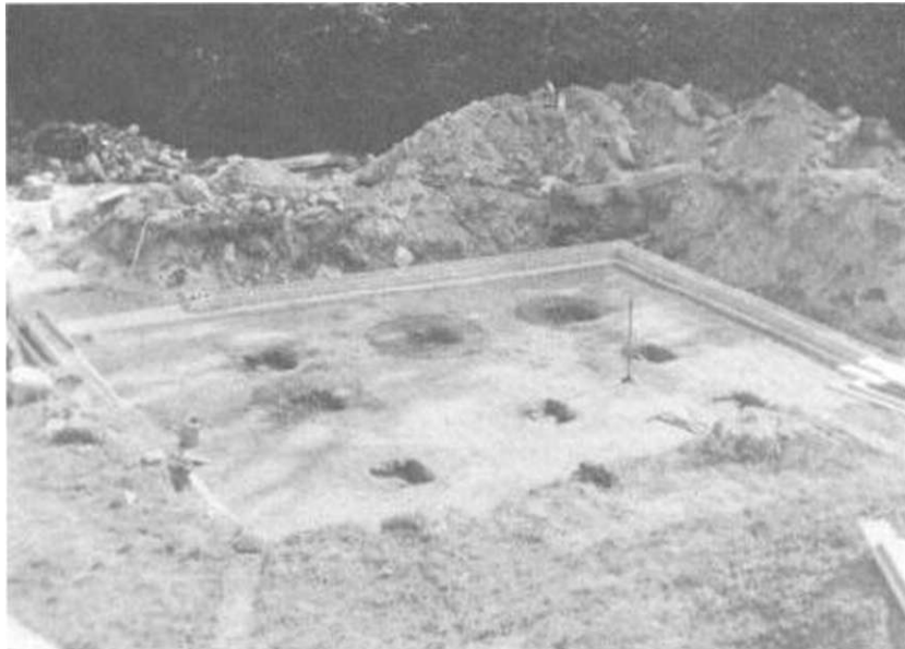
Illus. 5-5. The bottom half of the pillar footings can be poured at the same time as you pour the floor.
