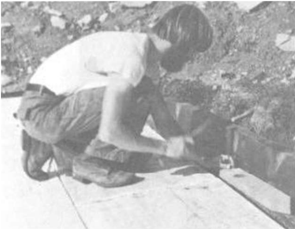
Illus. 8-8. fascia boards were fastened by first nailing a 2 x 6 plank along the edge of the roof then nailing a scrap piece of economy-grade 2 x 4s on top of the plank. These two pieces provide a base for fastening the 2 x 12 fascia.
