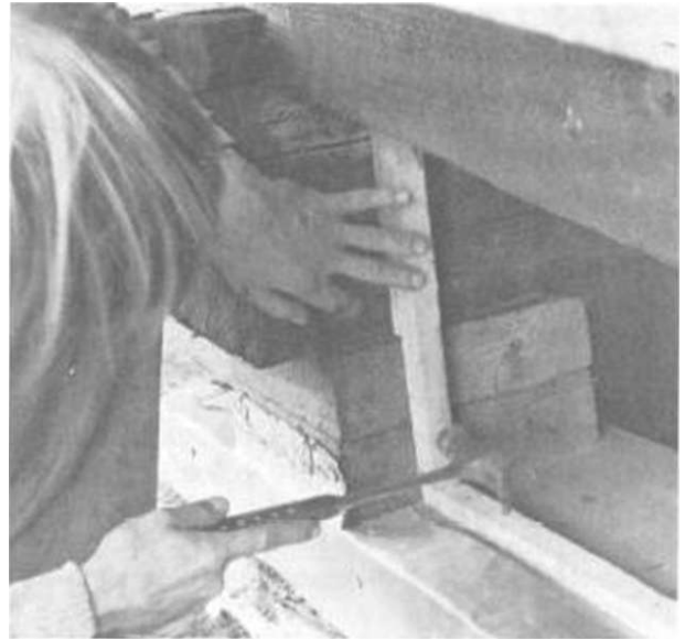
Illus. 12-3. Installing the trapezoidal window in the north wall. Since it was convenient to work from the outside, I fastened the inside molding first.
