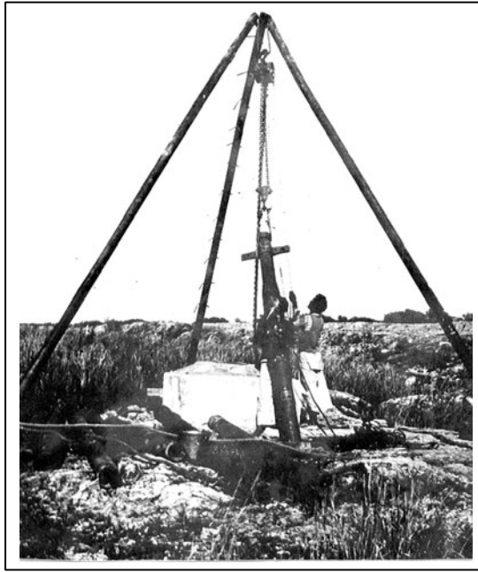
Fig. 11.20 Installation of a submersible pump in a tube well. The motor and pump assembly is being hoisted for lowering into the tube well
