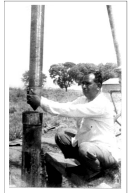
Fig. 5.58 Lowering a well screen into the casing pipe of well drilled with a percussion drilling rig
