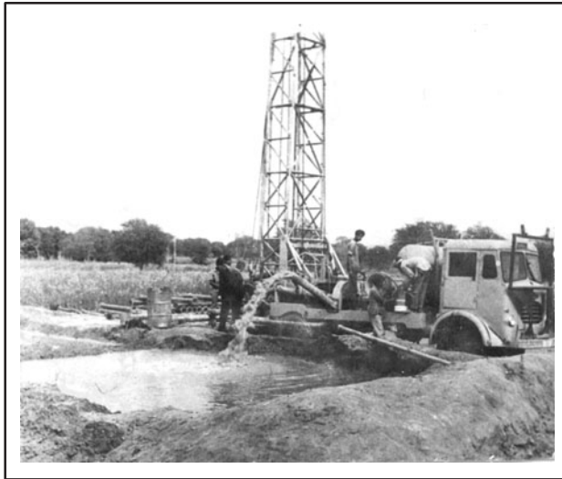
Fig. 5.32 Reverse circulation rotary drilling in progress. Note the water storage-cum-settling pit in the foreground
