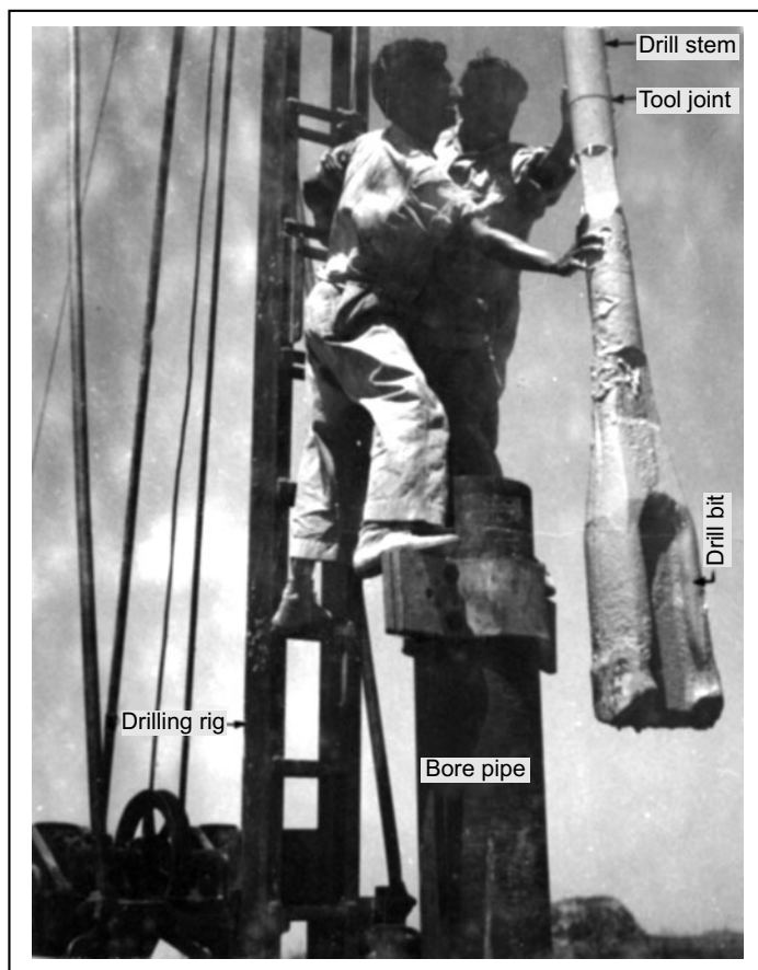
Fig. 5.6 Setting aside the drill bit before using the bailer in percussion drilling Courtesy: Television Kendra, Patna, Bihar
