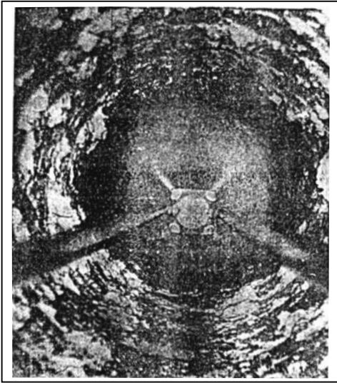
Fig. 7.5 Underwater view showing the inside of a screen tube well which is clogged by incrustation. Note the salt deposits blocking the slot openings of the well screen
