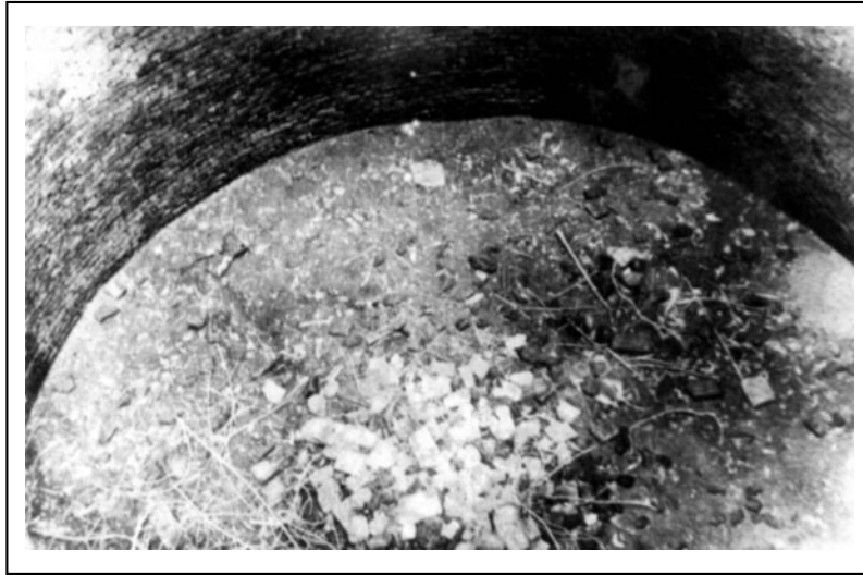
Fig. 3.30 An abandoned open well filled with garbage producing heavy pollution in the ground water in the surrounding region.
