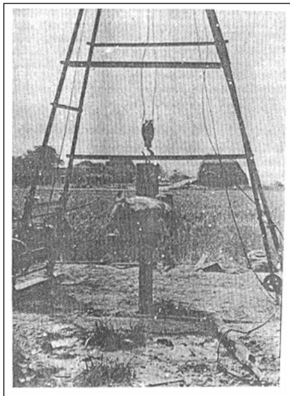
Fig. 5.19 Weighted drop hammer and sand bags used to drive in the outer casing pipe in cable tool drilling
