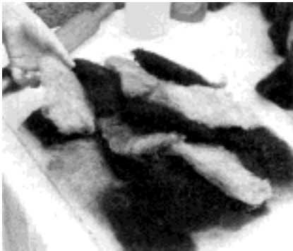
4. The third and fourth layers are laid over the first two layers. Notice the overlapping pattern.
