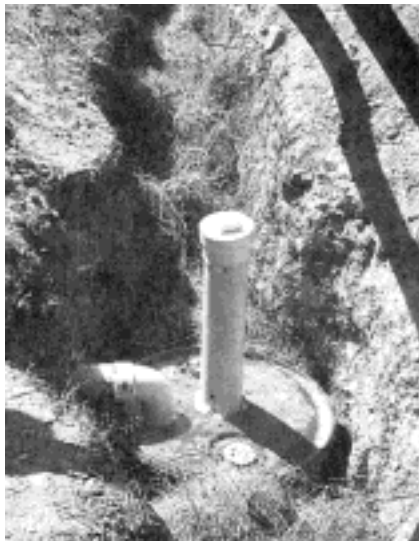
Tank with cleanout pipe mounted, hay in place, ready to be covered. Note generous amount of caulking around base of cleanout pipe.
