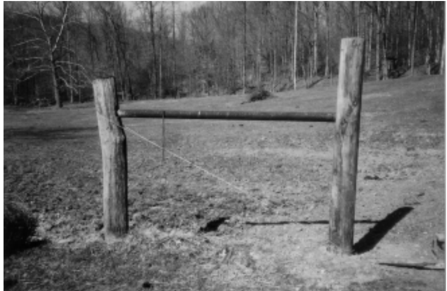
Properly set corner and brace posts. Note the diagonal brace wire runs from the base of the corner post to the top of the brace post. If a solid diagonal brace is used, run it from high on the corner post to the base of the brace post.
