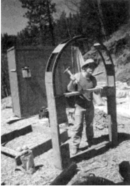
Framing for door opening. Blue air lock is visible in the background
