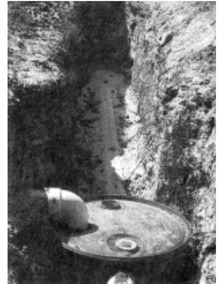
The tank is in the ground with gravel laid underneath the drain pipes. Use plenty of gravel for proper drainage.
