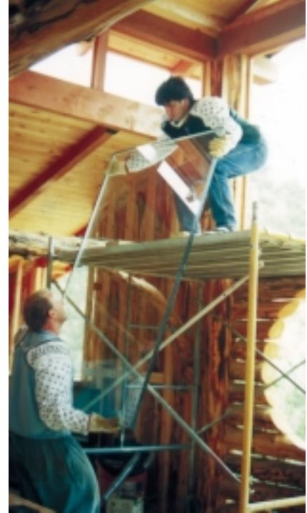
Vadim and Kirt, donning protective sleeves, handle heavy double-paned picture window glass.
