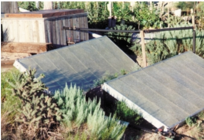
Tub with collector (lower right). Upper collector is for domestic water heating.
