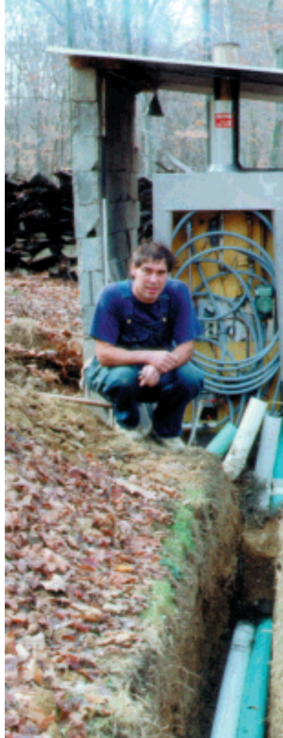
The stove sets on a concrete pad in a small shed. The trench connects it to the barn. The shed make it nicer when filling the stove in bad weather.
