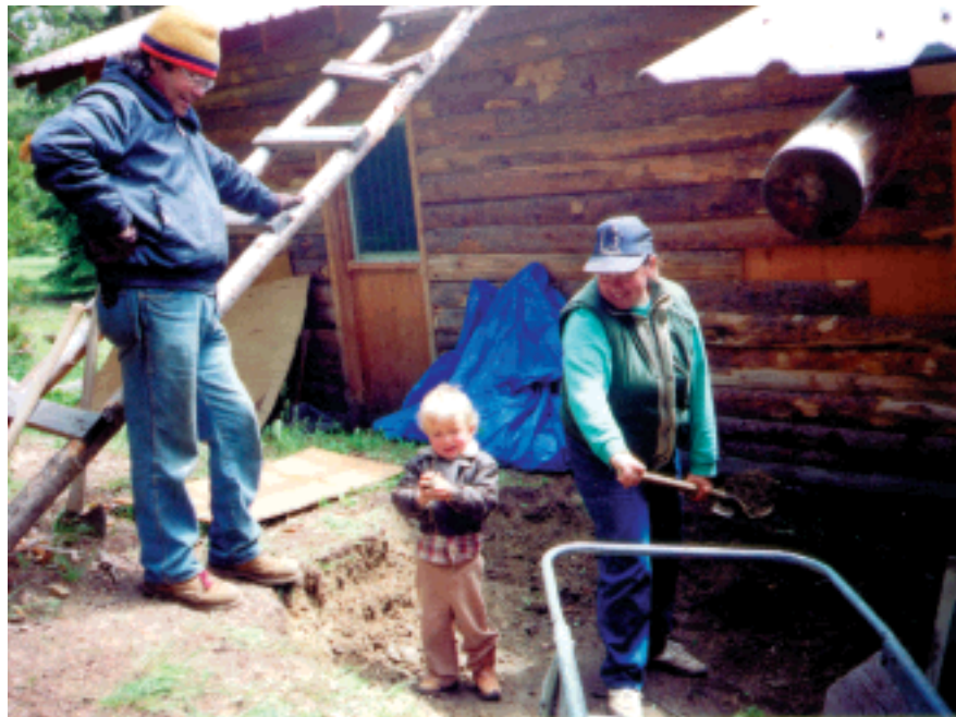
Digging out for the foundation of our new pantry addition to allow for two years of food storage
