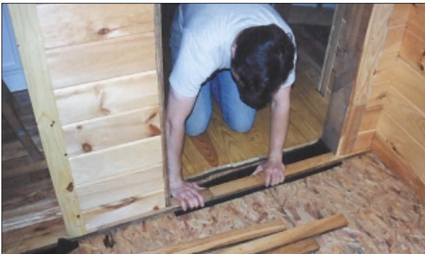
Fitting the oak flooring across a door opening requires patience and care.
