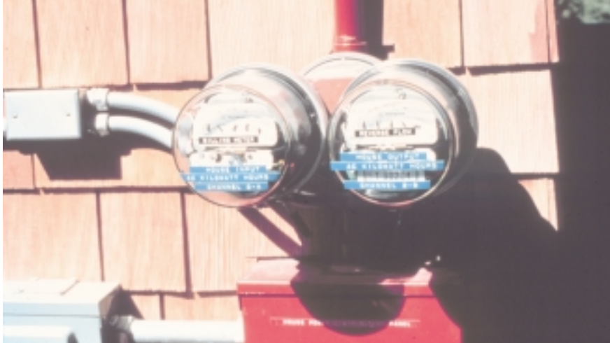
Dual meters are common when renewable energy systems put power back down the utility line.
