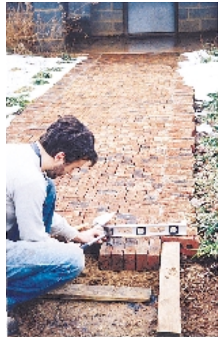
Figure 2. Lay a series of bricks, tap them down with the hammer, and level them. Notice the irregular exterior bricks that have already been mortared into place.
