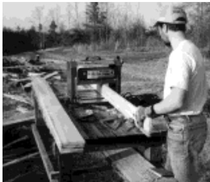
When we finished planing the wide surfaces, we stood the boards on edge and planed the edges.
