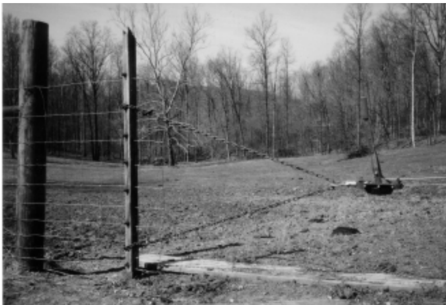
This photo shows how the wooden fence stretchers and “come-along” are used together. Notice how the wooden stretchers clamp tightly to the wire to help stretch the wire evenly.
