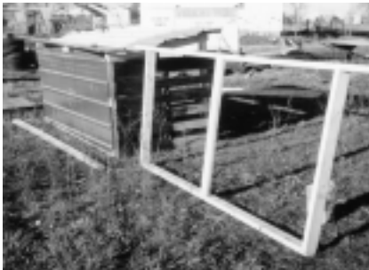
Figure 1. The basic frame for the front and back of the shed is in the foreground. The back is three and a half feet tall, while the front is four feet. This allows for water runoff.
