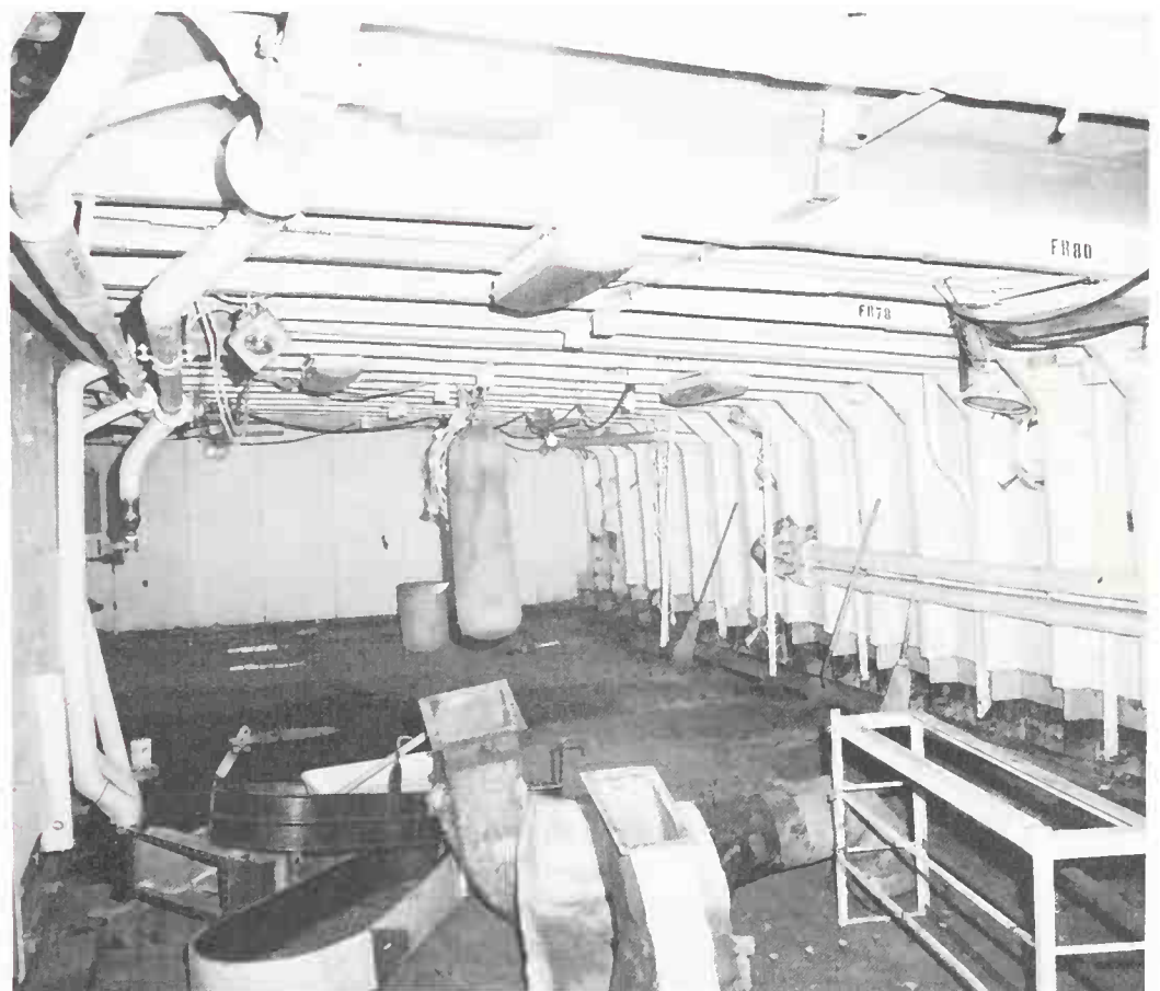
The new berthing area in an early stage during the great refurbishing. Nine new bulkheads were installed in these operations, bringing the ship up to full two-compartment status and modern standards of strength and safety. Notice the relatively light frames along the side of the ship. (U.S. Coast Guard photo)
