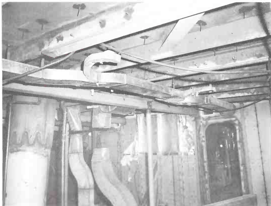
Ventilation conduits are installed during the great refurbishing of the early 1980s. (U.S. Coast Guard photo by Harry Butt)
