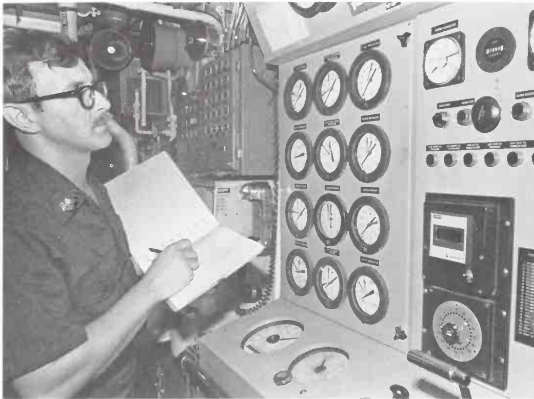
In the engine room, the engine's performance is read on dozens of gauges, every one of which is checked and logged at the beginning and the end of every engine-room watch. "Max," the 1000-horsepower main drive plant, dominates the engine room. (U.S. Coast Guard photos by Doug Bandos [top] and Paula Hobson)
