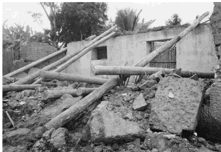
Figure 2: The impact of the earthquake on a tapial house in Soritor © Practical Action/Megan Lloyed-Laney
