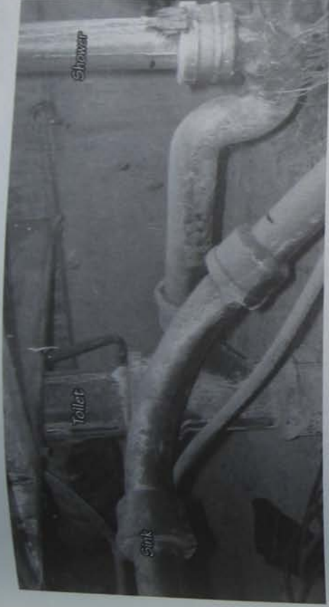
Before: cast iron drain pipe for a bathroom in an old adobe home in New Mexico.
