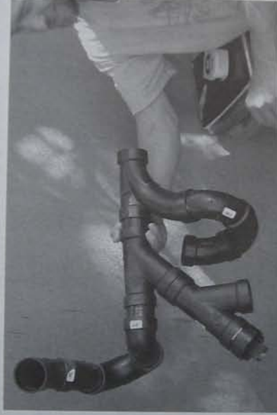
Greywater plumbing subassembled (no glue).
