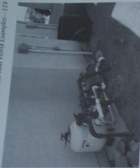
ReWater surge tank, sand filter.
