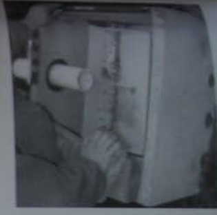
Leveling a dipper. Stand on it and wiggle it down into the concrete while checking for level in both directions.
