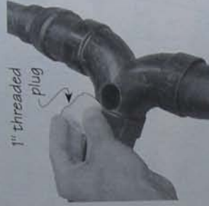
A double ell retrofitted with inspection access. The access is sealed with a threaded plug. 69
