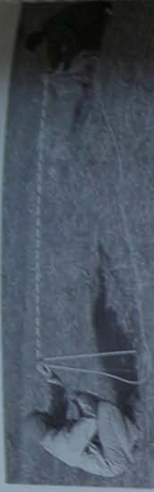
Checking levels with a water level. Person at right adjusts tube until water level is at her reference mark. Person at left measures from water level to top of ground.
