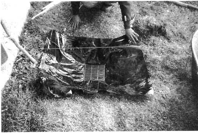
Fig. 4.7A. Pond liner and drain box with the X-cut in the plastic beneath the grate so water can freely drain into the drain box. Credit: Jeremiah Kidd
