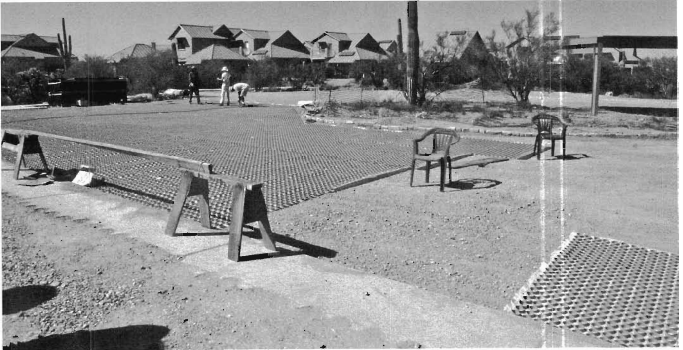
Fig. 8.17A. Gravelpave 2 geocells with landscape fabric backing being installed at Milagro Cohousing parking lot, Tucson, Arizona. Flush concrete curb will strengthen the edge between the geocell surface and the incoming stabilized-earth road.
