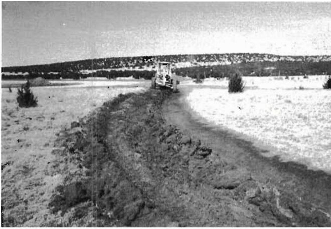
Fig. 9.21. Grader cutting diversion swale on Chris' land. Note: The operator was not allowed to drive grader on the downslope side of swale in order to retain all soil-stabilizing vegetation over which swale overflow water would flow. Credit: Chris Meuli
