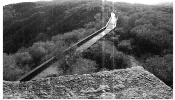
Fig. 9.10B. Diversion swale entering the Jaipur Fort (foreground), and the 2.4-mile (4-km) catchment in the background
