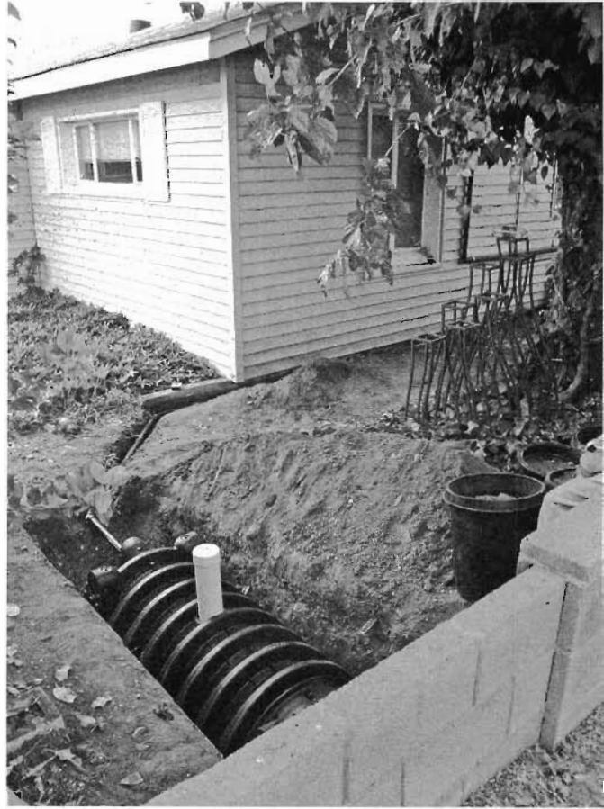
Fig. 12.12A. A premanufactured Infiltrator Systems outlet chamber sized to handle the peak surge of greywater entering the system from a bathroom sink. The soil percolation rate is slow due to high-clay soils. Urban Farm, Phoenix, Arizona. Note: These infiltration chambers also work great for septic leach fields, since you can plant trees beside them to utilize the “waste water.”
