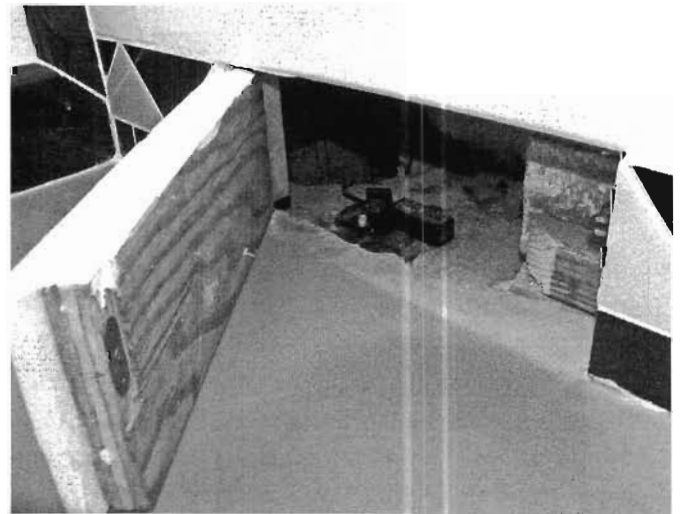
Fig. 12.7B. Closeup of bathtub diverter valve. Credit: Sonya Norman. For more stub-out examples see the Images page at www.HarvestingRainwater.com
