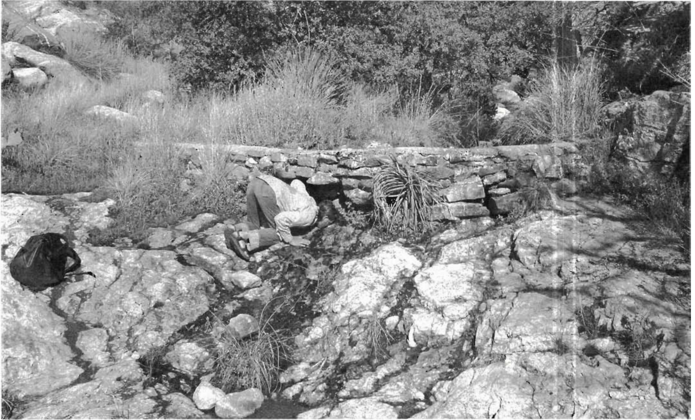
Fig. I.11. A check dam built long ago atop bare bedrock has accumulated, upslope of the dam, a level terrace of soil and organic matter in which vegetation now thrives. The harvested soil and organic matter act as a sand tank that quickly infiltrates stormwater flow, then slowly releases it to the plants' roots, and as a seeping flow over the bedrock that continues to run for weeks after the last rain. Anastasia Rabin enjoys a drink of this tasty water. Pima Canyon, Tucson, Arizona. For color photo see inside front cover.
