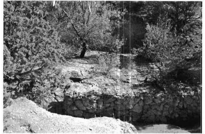
Fig. 10.15. Poorly built gabion with a flat top and no low center or bank protection. Flowing water was spread to the banks where it cut around the gabion at the left, so the soil has eroded.
