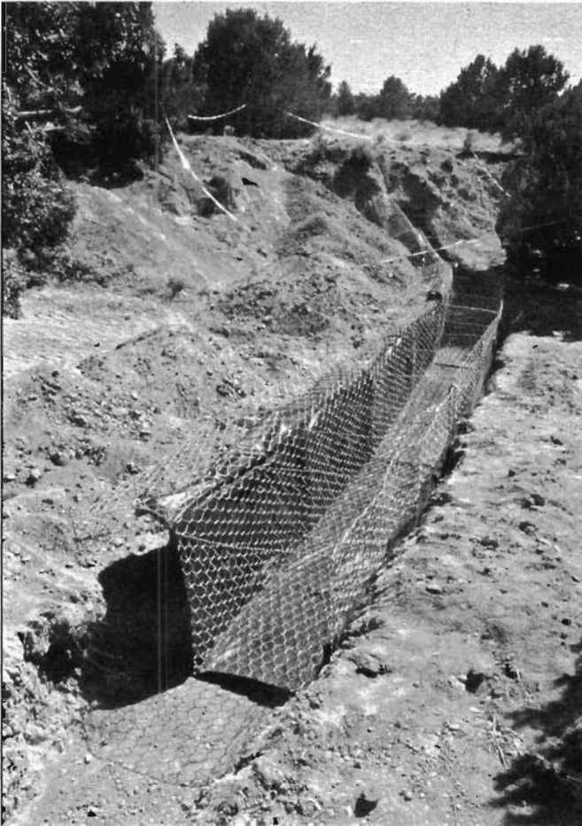
Fig. 10.14. Gabion baskets lined with landscape fabric being laid in a trench sloping up the banks. Landscape fabric and excavated dirt are on the upslope side of the basket. Note that the basket top is folded open to the upslope side, so when it is folded closed it will be folded in the direction of water flow. Compare to figure 10.22, which shows the finished gabion.
