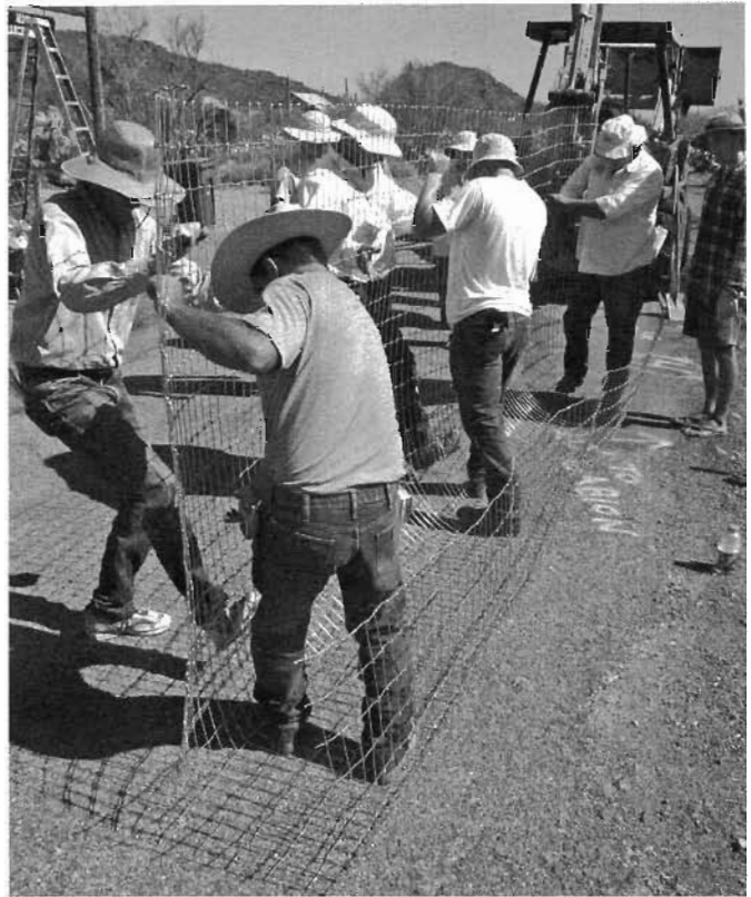
Fig. 10.16. Bending fencing into a gabion basket. Two lengths of fencing were first overlapped and hog-ringed together to make a larger basket. The longer side of the basket will go on the upstream side of the trench so it can later be folded downstream to cover the top of the rock that will be placed within the gabion basket. Excess fencing can be cut off once the rocks are placed within, and fully wrapped by, the basket.
