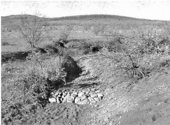
Fig. 10.29A. One-rock dam, Red Windmill Draw, Malpai Ranch, near Douglas, Arizona. Reproduced with permission from An Introduction to Erosion Control by Bill Zeedyk and Jan-Willem Jansens. Photo credit: Van Clothier
