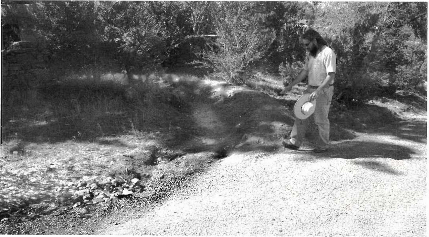
Fig. 9.8. A diversion swale that diverts runoff from a driveway-side drainage ditch into existing vegetation. The swale bends and levels, terminating as a contour berm. Work by San Isidro Permaculture and Raincatcher. Santa Fe, NM.
