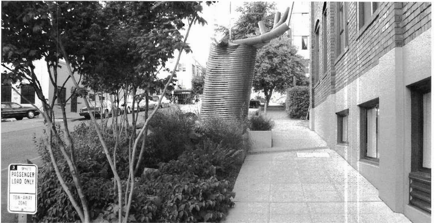
Fig. 3.21. The Beckoning Cistern and terraced planters. This 10-foot (3-m) high, 6-foot (1.8-m) diameter metal culvert cistern/sleeve reaches upward, capturing roof runoff through the hand's index finger and sending overflow out its thumb. The overflow water is then caught by a series of terraced planters. Terrace walls double as seating benches.
