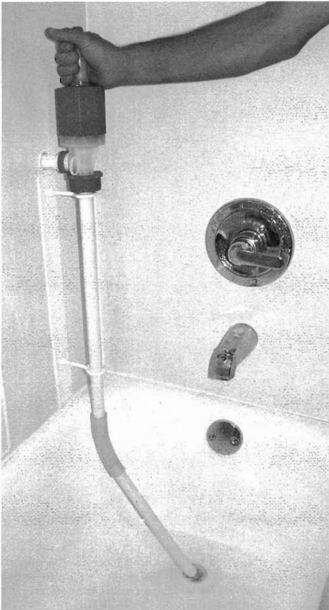
Figure 12.17A. The hand pump siphons the tub's greywater through a rigid intake pipe, up to the pump, then through a hole bored in the exterior bathroom wall, carrying greywater out to mulched and vegetated basins located outdoors. The type of rubber drain screen that has a depressed cup to catch hair, but allows water to pass through, is adapted for use as the intake point for the pump pipe by sealing the screen holes with white silicone caulk (see fig. 12.18). The adapted drain screen prevents the tub from draining and constitutes the lowest point in the bathtub. The tip of the pump's intake pipe is set at this low point to suction water from the tub.
