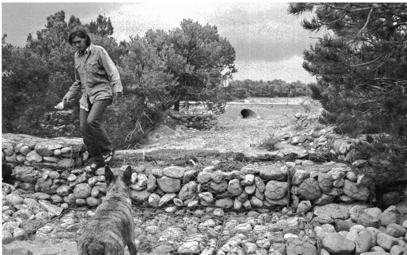
Fig. 10.3. Gabion stabilizing erosion caused by upstream culvert. Work by Santa Fe Permaculture
