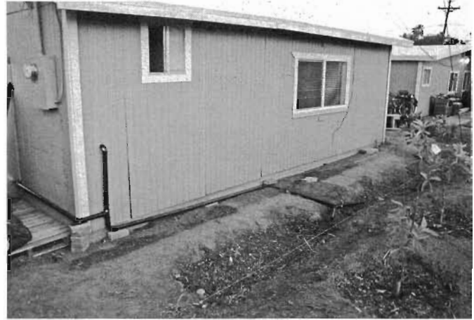
Figure 12.17B. The vertical pipe conveys greywater siphoned from the bathtub (Note: For the siphon effect to work, the hand pump's corrugated outlet tubing must run through the wall then downward inside the exterior plastic pipe until it exits below the bottom elevation of the tub). The horizontal pipe rounding the corner of the house conveys gravity-fed greywater from the bathroom sink's three-way valve (see fig. 12.6), then the 1.5-inch (40-mm)-diameter ABS plastic pipe directs this greywater to mulched basins via a branched-drain system. While the system is under construction, the horizontal greywater pipe is supported by bricks in preparation for attaching the pipe to the wall with brackets. Basin edges will be stabilized with rock and the basins will be planted.
