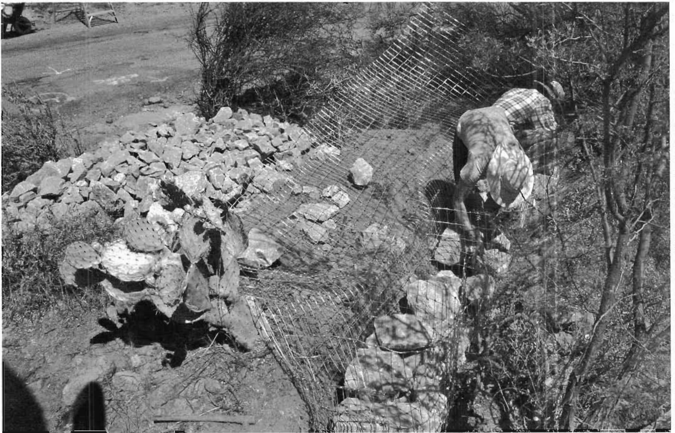
Fig. 10.18. Setting rock within a homemade gabion basket. Angled rocks are set firmly in place, with the larger rocks placed at the bottom, and the flat faces of large rocks facing outward for a neater appearance. Smaller rocks can then fill the core of the gabion. The basket lid is temporarily weighted down with rock so gabion builders can walk over it as they step in and out of basket. Direction of water flow is from left to right, so gabion will help stabilize once-eroding road. The entire pile of rock will be used within the gabion basket and its apron.
