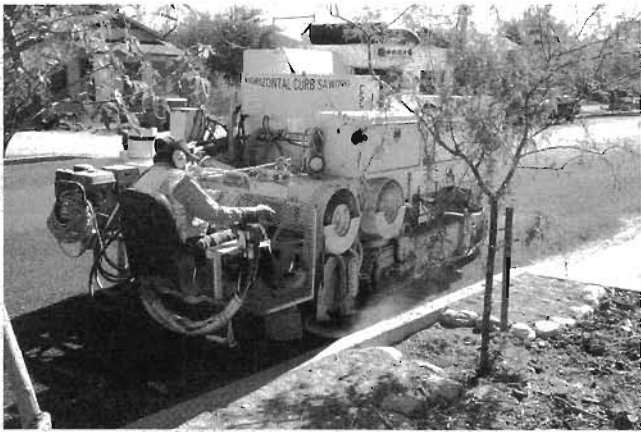
Fig. 8.35A. Concrete-cutting service beginning to make the horizontal cut of the curb cut
