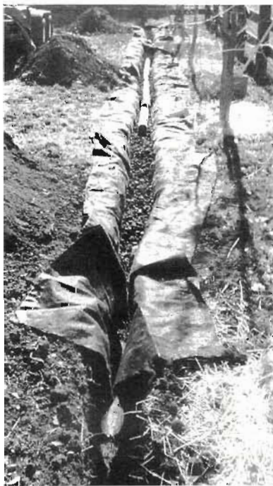
Fig. 4.9A. Perforated pipe being laid level within a French drain of gravel wrapped in landscape fabric. The French drain will direct roof runoff to passively irrigate a windbreak of trees. Credit: Jeremiah Kidd
