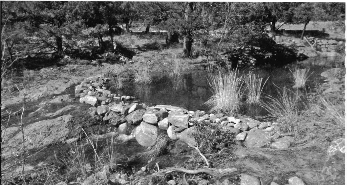
Fig. 10.39. Turkey Pen watershed check dam. There is no apron since the dam was built atop bedrock. Note the flat top of the dam. This has led to end cutting on some of the dams, which could be avoided if the center of the dam were made lower and the ends higher to direct overflow down the middle of the drainage while protecting the banks.
