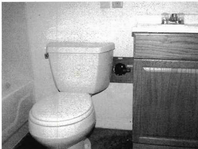
Fig. 12.6. Three-way diverter valve conveniently located between toilet and sink directs sink greywater to landscape or sewer at the Eco Hood in Phoenix, Arizona
