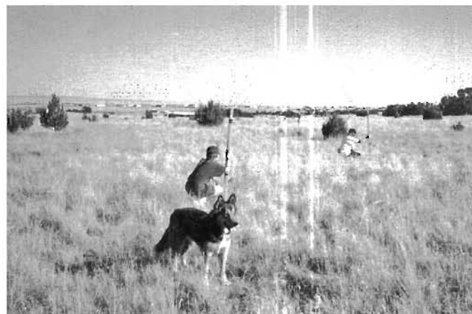
Fig. 9.19. The first step in laying out a spreader drain: Chris Meuli's young neighbors (and their dog) bunyip a contour line across a 3% slope on Chris' property. Credit: Chris Meuli
