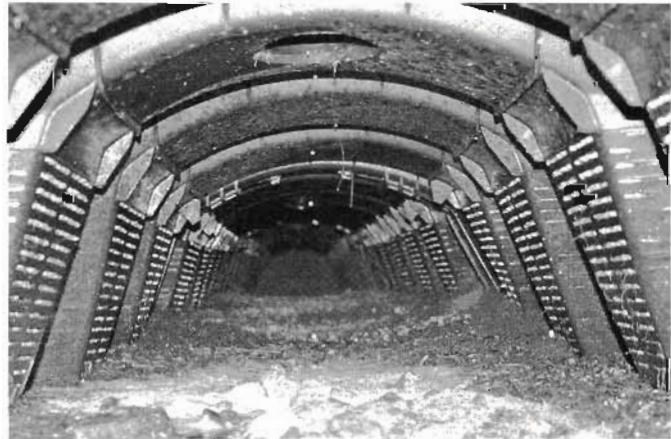
Fig. 12.12C. The interior of three Infiltrator Systems infiltration chambers linked together, Lama, New Mexico.
