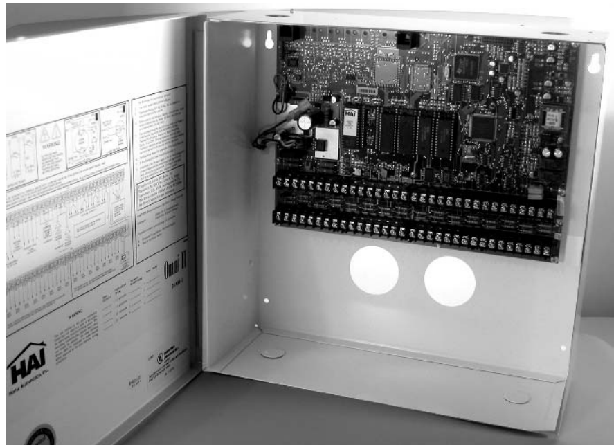
Figure 5-1 Omni II control panel
