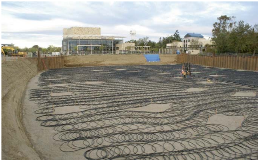
Fig. 7.4 Construction of geothermal ground loop system to provide heating and cooling (Credit: Bovis Land Lease)
