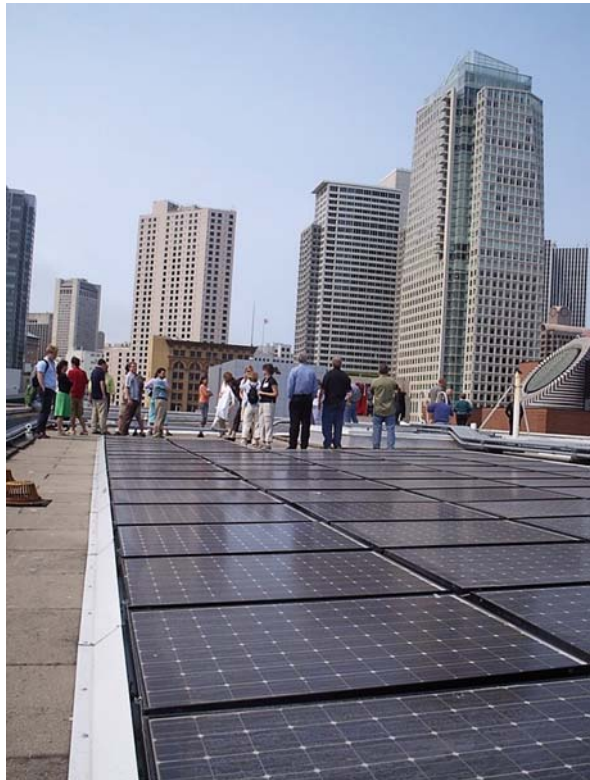
Fig. 7.2 Solar panels on the roof of the Moscone Center
