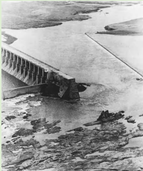
The concrete structure of the Manchu River Dam in Morvi, India. AP IMAGES.
