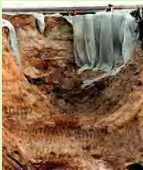
Heavy rains from an El Niño-driven storm caused this 65 foot sinkhole in Balboa Avenue in San Diego, California.
