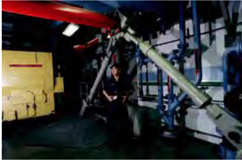
Earthquake braces installed at Diablo Canyon nuclear power plant in California. ©ROGER RESSMEYER/CORBIS.
