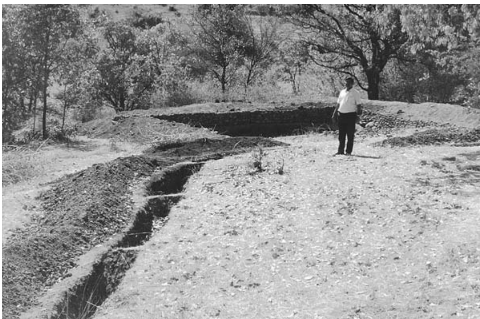
FIGURE 7 Contour bund with contour trench and farm pond on upslope side Near road between villages of Manhere and Ambevangan, Akole Taluka , Ahmednagar District, Maharashtra State, India.
