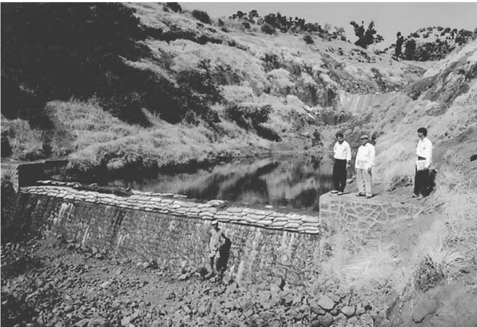
FIGURE 5 Lowermost check dam and reservoir in gravity-flow system of three reservoirs, close to completion Middle and uppermost check dams of system also visible. Near Manhere Village, Akole Taluka , Ahmednagar District, Maharashtra State, India.
