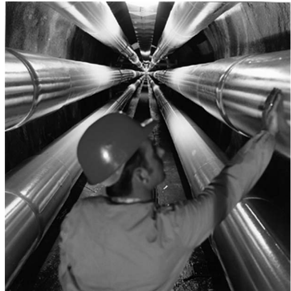
Figure 9. View into the tunnel with a double system of single-phase GIL.
