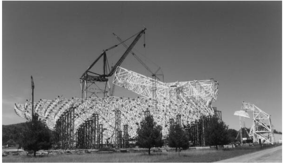
Figure 12. Construction site of the Green Bank Radio Telescope reflector antenna. The 100 m main reflector consists of 2000 solid panels. The structure can be pointed to view the entire sky down to a 5^\circ elevation angle and will be the largest fully steerable radio telescope in the world. (Courtesy of George Behrens, National Radio Astronomy Observatory.)
