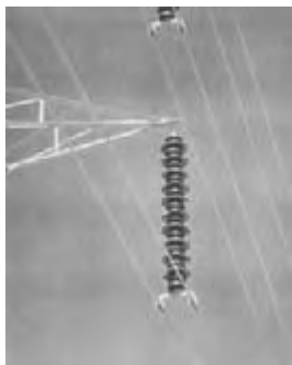
FIGURE 5.7 Creepage Extenders Installed in a Transmission Line. Courtesy of Tyco Electronics.
