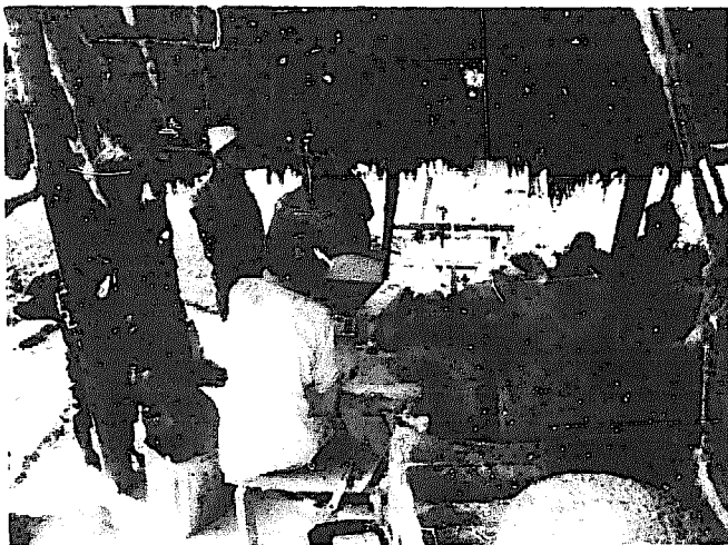
Front view of the same installation: the power take-off (axle with three pulleys) transfers the power of the turbine (top most pulley) to the rice huller and/or grinder.
