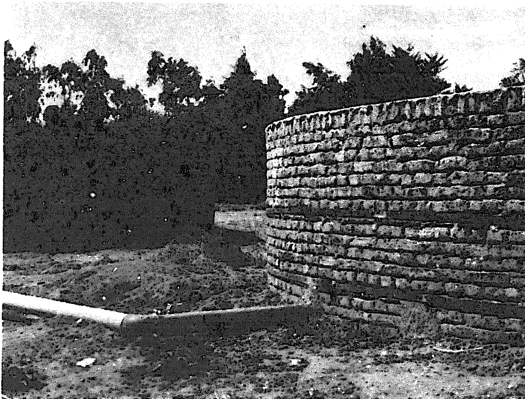
A storage tank adds considerably to the costs of a pumping system. The tank on the left has cracks in the outer wall. The tank on the right has been reinforced with steel straps.
