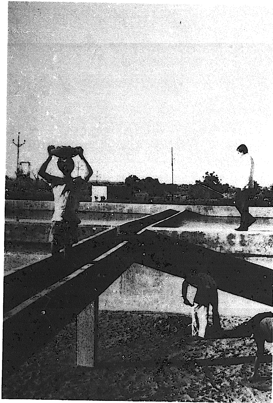
Figure 15.12. Manual cleaning of a slow sand filter
