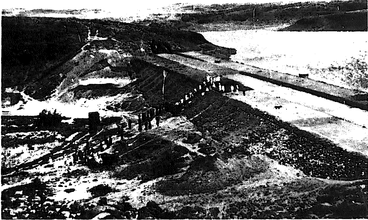
Fig. 10. Percolation dam being built in the Maharashtra state of India, December 1969. Construction was by manual labour paid for on a food-for-work basis.
