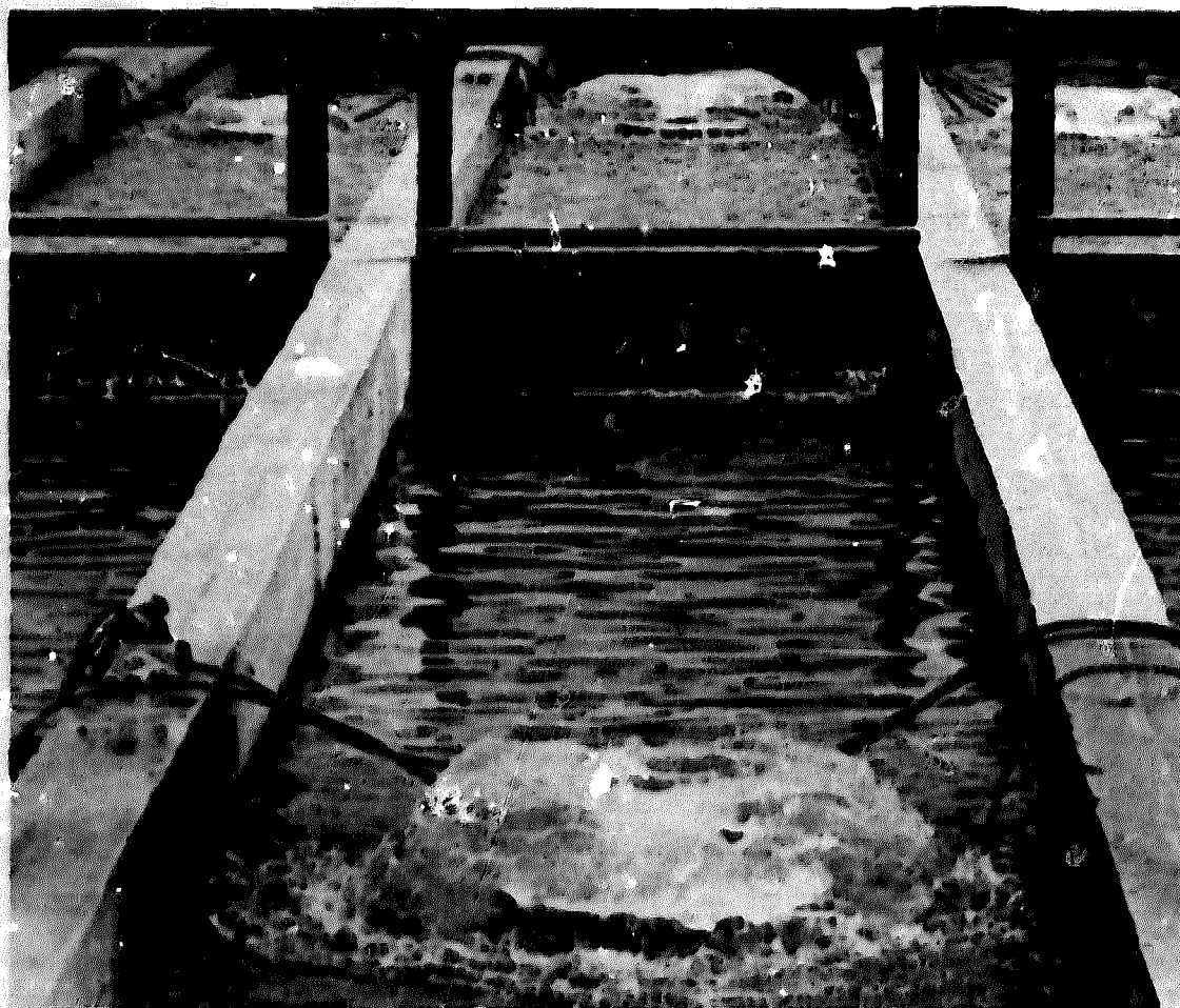
Through forceful mixing action a surface aerator speeds the migration of oxygen molecules from air to water.
