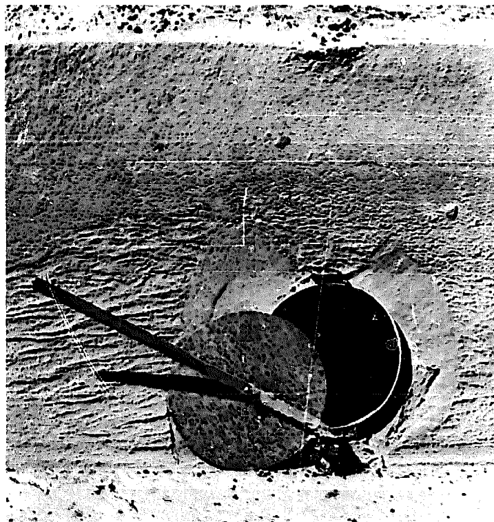
FIGURE 62. Circular gate on pipe outlet from concrete-lined canal.
