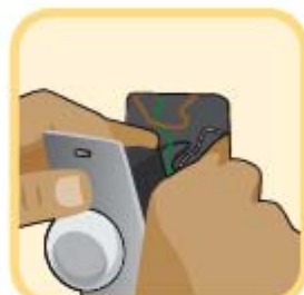
Fold the wires back into the box.
