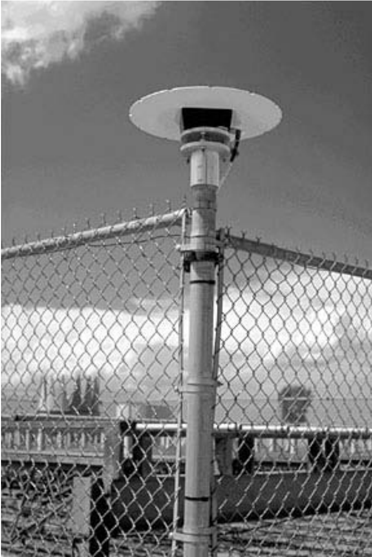
Figure 6. GPW-IPW installation at the NOAA Profiler Network site at Platteville, Colorado.
