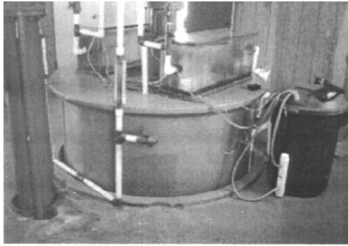
(Long beach facilities showing control tank (left) and magnetically treated water tank (right) with nutrient feeding tank)
