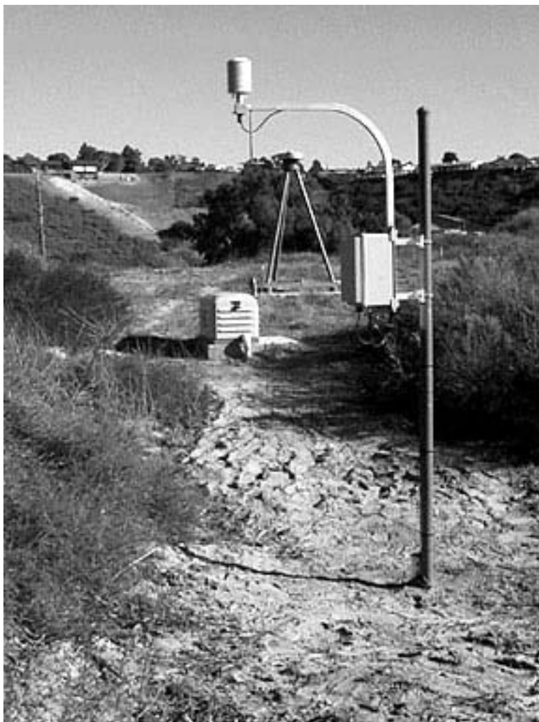
Figure 7. GPS-IPW installation at the Scripps Institution of Oceanography at La Jolla, California.
