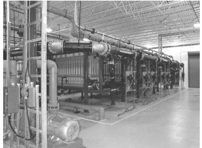
Figure 3. Microfiltration (MF) system (Source: U.S. Filter).
