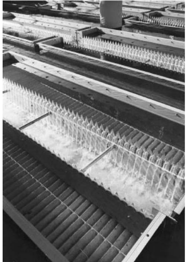
Figure 4. Installed plate settlers (Source: U.S. Filter).
