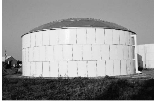
Figure 1. Ground-level water storage tank (Source: Columbian TecTank).
