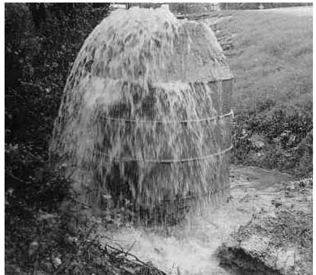
Overflowing sewer due to a sewer blockage
