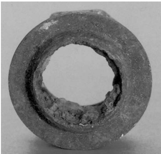
Figure 1. The cut section of a cast-iron pipe shows a severe iron bacteria buildup on the pipe walls.
