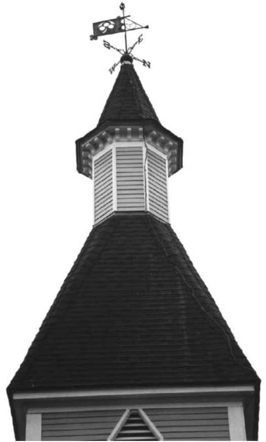
Figure 2. A weathervane and lightning rod combination. Location: Trinity Methodist Church, Oak Bluffs, Massachusetts (photograph courtesy of William Waterway).
