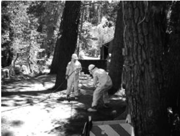
Figure 1. Handheld lances used to perform remediation by jetting technology in a limited-access site (FAST-TEK).
