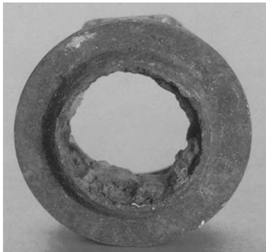
Figure 3. The cut section of a cast-iron pipe shows a severe iron bacteria buildup on the pipe walls.
