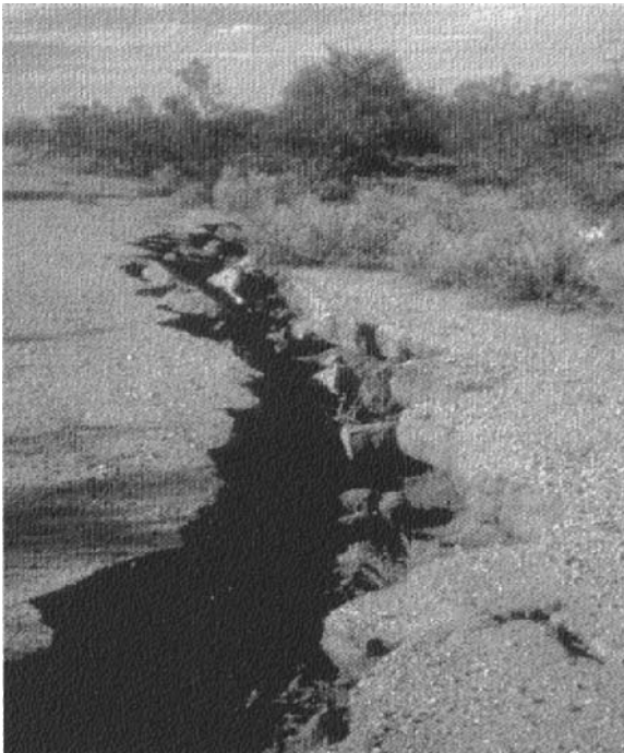
Figure 2. Pima County, Arizona. Sign warning motorists of subsidence hazard was erected after an earth fissure damaged a road in Pima County, Arizona (left photograph). Earth fissure near Picacho, Arizona (right photograph) (photographs by S.R. Anderson, U.S. Geological Survey).
