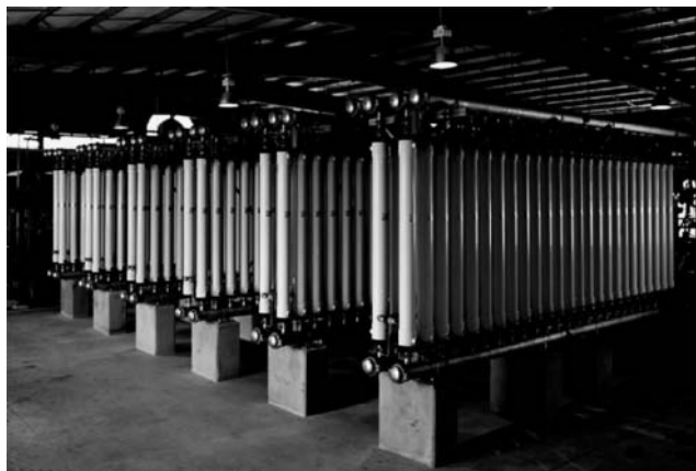
Figure 4. Membrane filtration system (Source: PALL).
