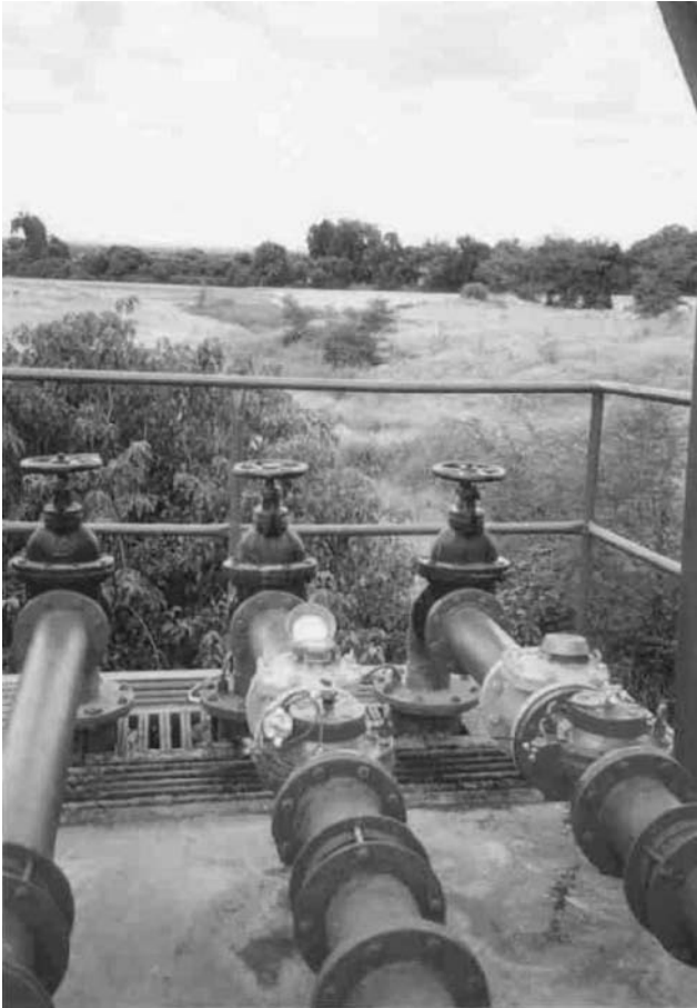
Figure 5. Submersible pumps drawing water for a commercial irrigation scheme from the sand of the Limpopo River in the background.
