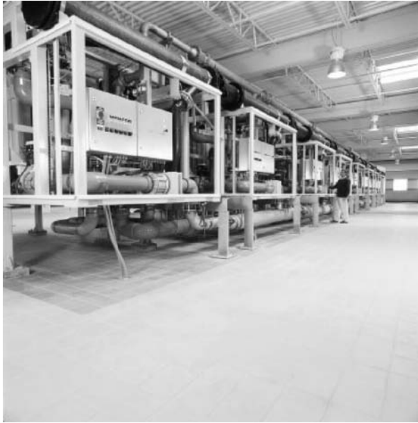
Figure 4. Microfiltration (MF) system (Source: U.S. Filter).
