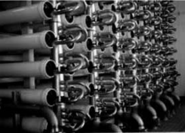
At West Basin Wastewater Treatment Plant in California, reverse osmosis, an advanced treatment process, is used to physically and electrostatically remove impurities from the wastewater.
