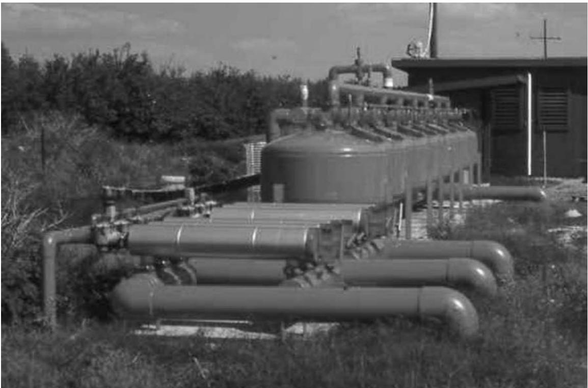
Figure 2. Media filters installed in a field.
