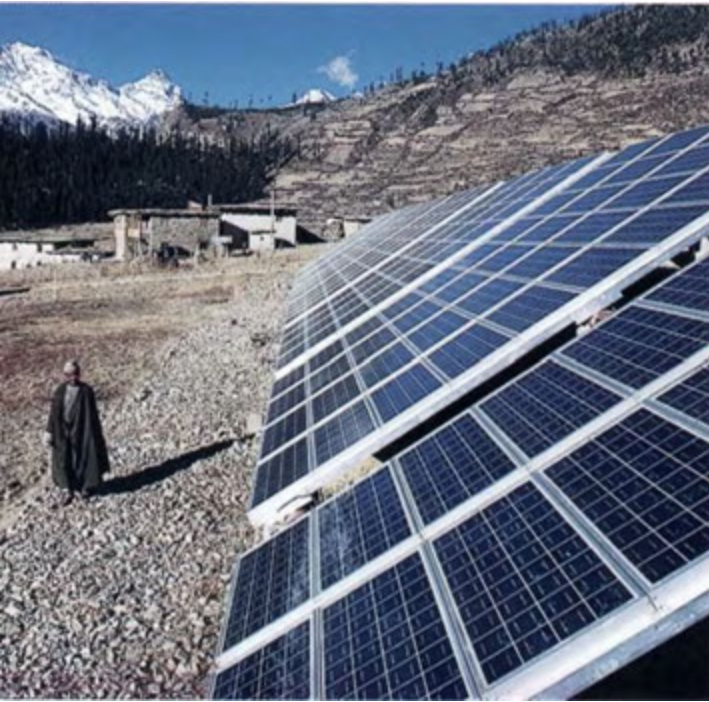
Figure 23.16 Solar cells convert sunlight, a renewable resource, into electric energy at this utility in a remote village in Nepal. [Ned Gillette/Corbis.]
