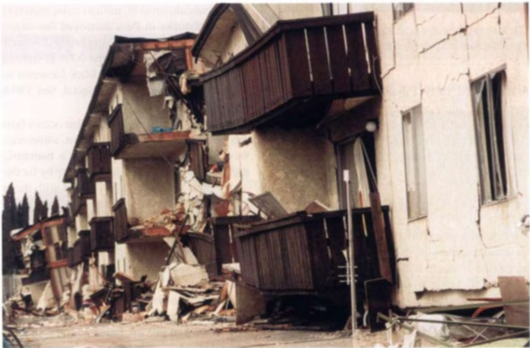
Figure 13.14 Sixteen people died in the Northridge Meadows apartment building in Los Angeles during the 1994 Northridge earthquake. The victims lived on the first floor and were crushed when the upper levels collapsed. Many more buildings would have
