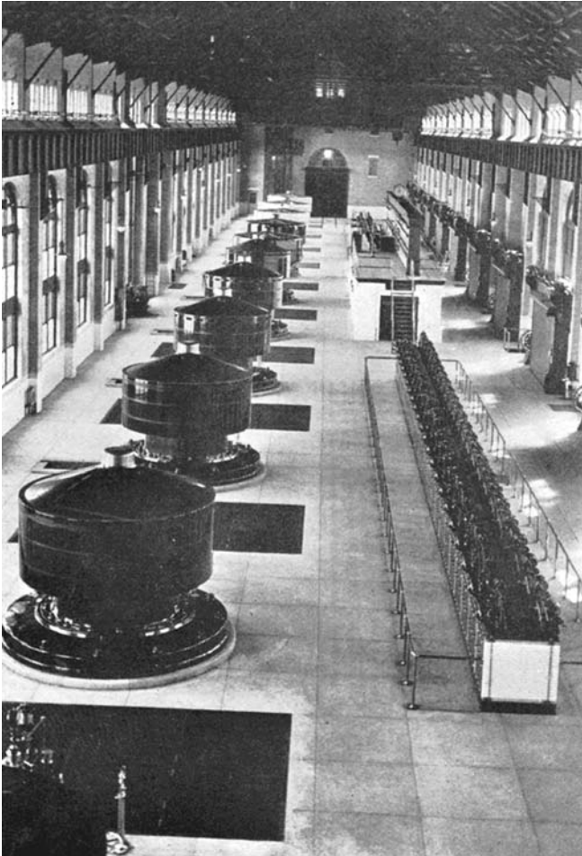
INSIDE THE NIAGARA FALLS POWER HOUSE NO. 2 The first Niagara Falls Power House was built between 1892 and 1894, opening for business in 1895. Its immediate success brought industry into the Buffalo region and Power House No. 2 was built between 1901 and 1903. Other generating facilities were built around the same time, each collecting some of the energy from the Falls and converting it to electricity.
