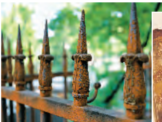
An untreated iron gate will rust.
