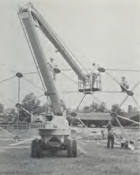
354 Giraffe crane speeded erection of 114-foot Geodesic pavilion at Winthrop Rockefeller's Winrock estate, Hot Springs, Arkansas, 1956.
