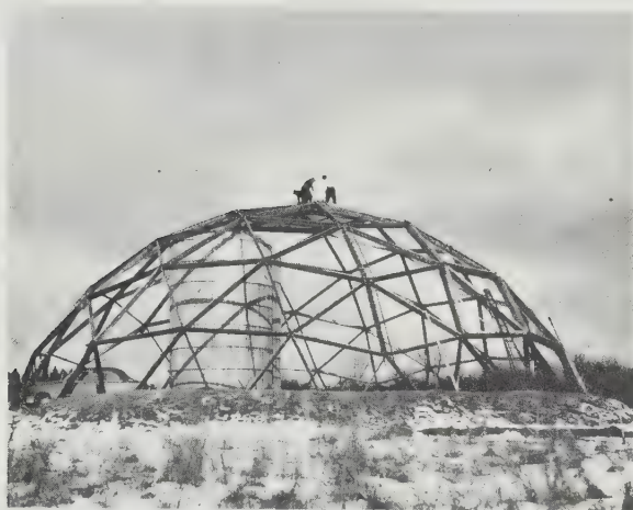
349 Laminated wood strut, polyester Fiberglass skin dome, 85 feet in diameter, built by Jeffrey Lindsay to be used as a barn, Montreal, 1954.
