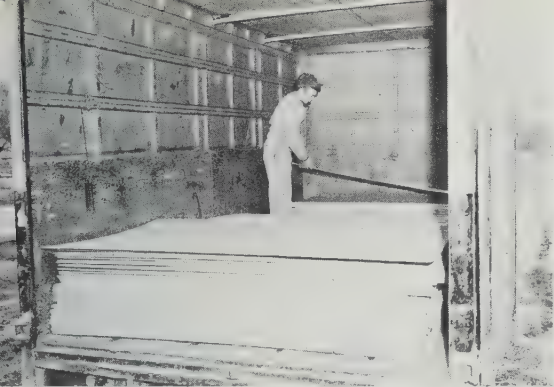
437 All the printed and punched \frac{1}{4} -inch Plywood components for a 42-foot dome arrive at site.
