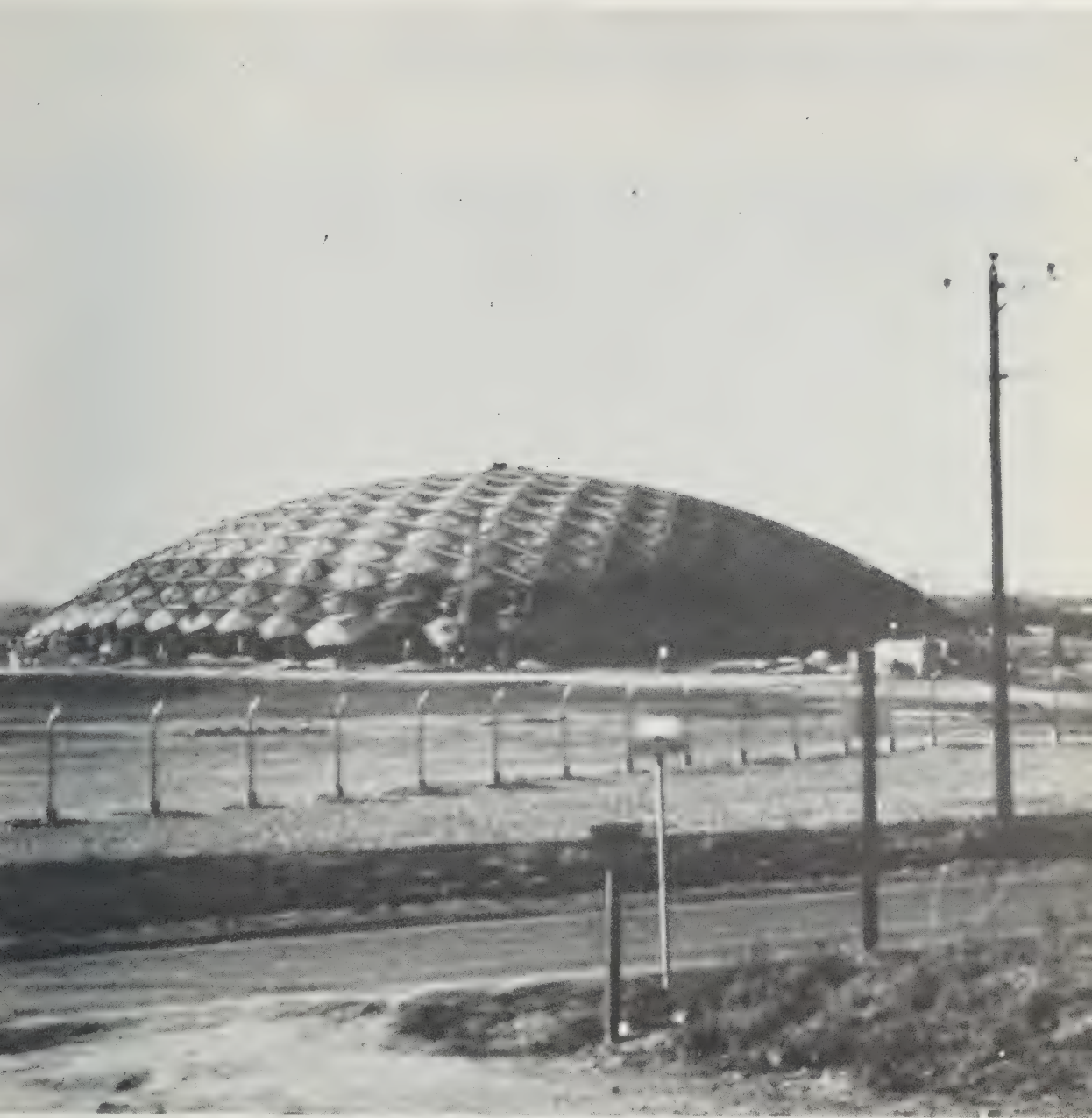
484 Union Tank Car Company's second Geodesic, 354 feet in diameter, marketed by their Graver Tank Division, as the "Union Dome," under erection by pneumatic cushion lift, at Wood River, Illinois, winter, 1958-59.
