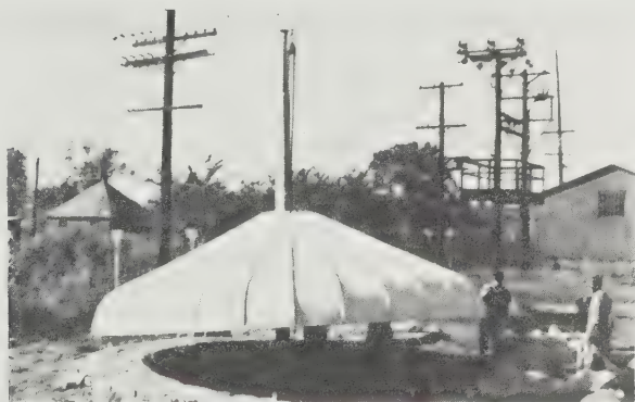
172 Similar to Fuller's Dymaxion 4D house, the D.D.U. was always erected from the top down. The roof parts were assembled on the ground and hoisted aloft. The body sheets were installed at a comfortable working height for workmen standing on the ground, and were hoisted in consecutive tiers. Butler's conic grain bin roofs could not be elevated in this manner because their straight line joints acted as hinges. One panel would hinge out as another hinged in, as gravity forced a hoisted conic top into a pleated-skirt. The curved joints of Fuller's compound eaves prevented such hinging. The wider the radius, the more the curvature, and the less the local effort required to maintain structural stability. (1940)
