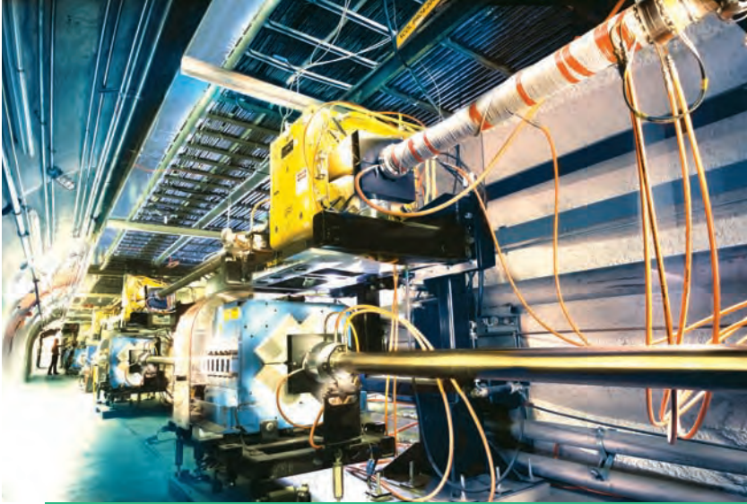
These pipes carry beams of particles in an accelerator at SLAC. ( Stanford Linear Accelerator Center )
