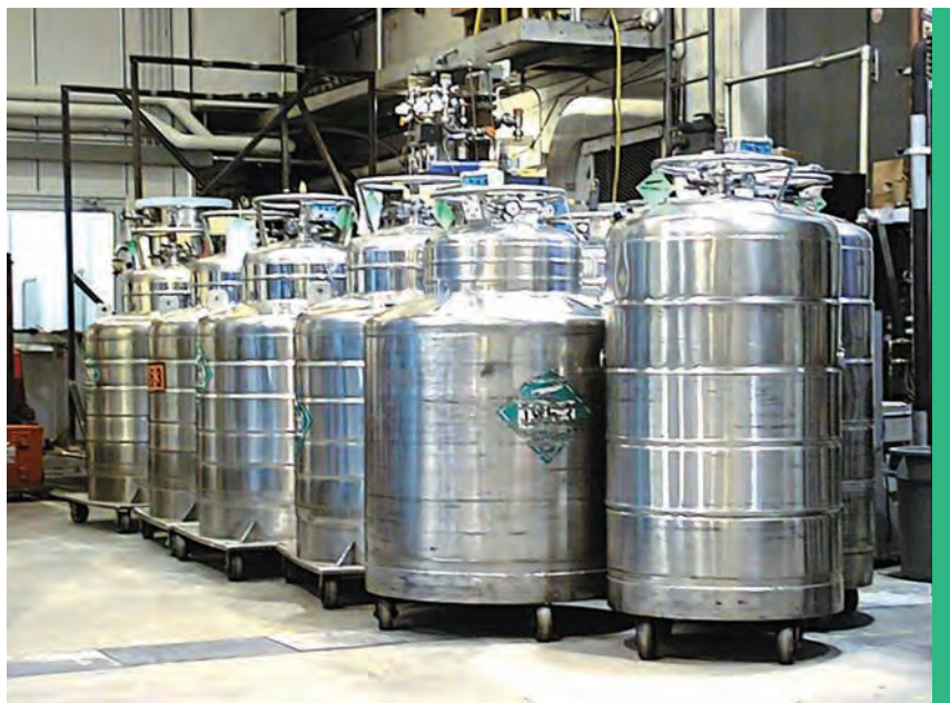
Insulated containers of liquid helium (Cornell—LEPP)
