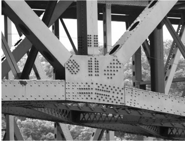
FIGURE 12.7 Joint Formed by Riveting a Gusset Plate to Converging Members (Used with Permission of Landov Media, New York)
