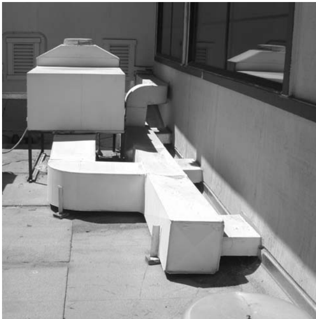
Fig. 11 A poorly installed IDEC system. The ductwork is far too restrictive to deliver the airflow needed to meet the cooling requirements of this classroom. Source: From Sacramento Municipal Utility District (see Ref. 7).
