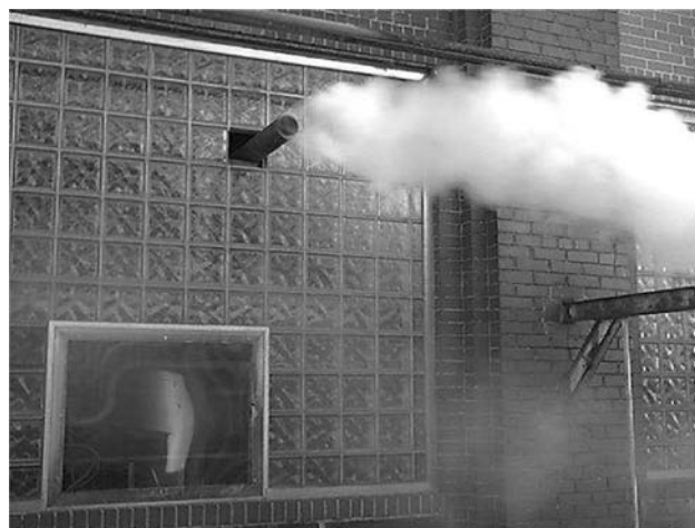
Fig. 6 Leaking relief valves vent.
