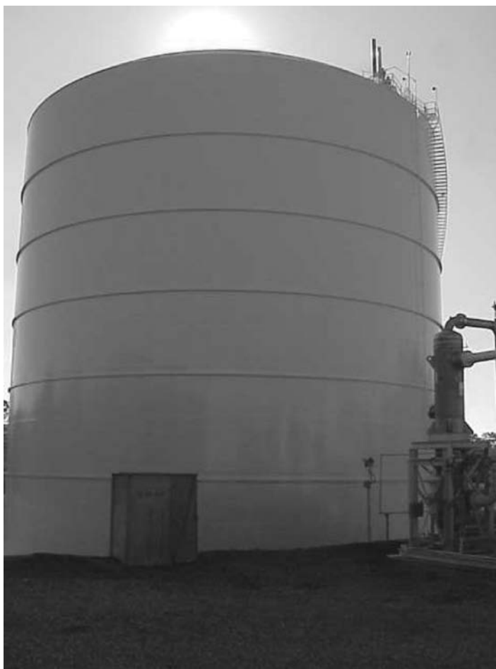
Fig. 3 Liquefied natural gas (LNG) storage tank with remote heat vaporizer in right foreground. Note relief valve stacks on tank top.
