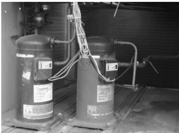
Fig. 3 Two-compressor HVAC package unit where one compressor was not needed.
