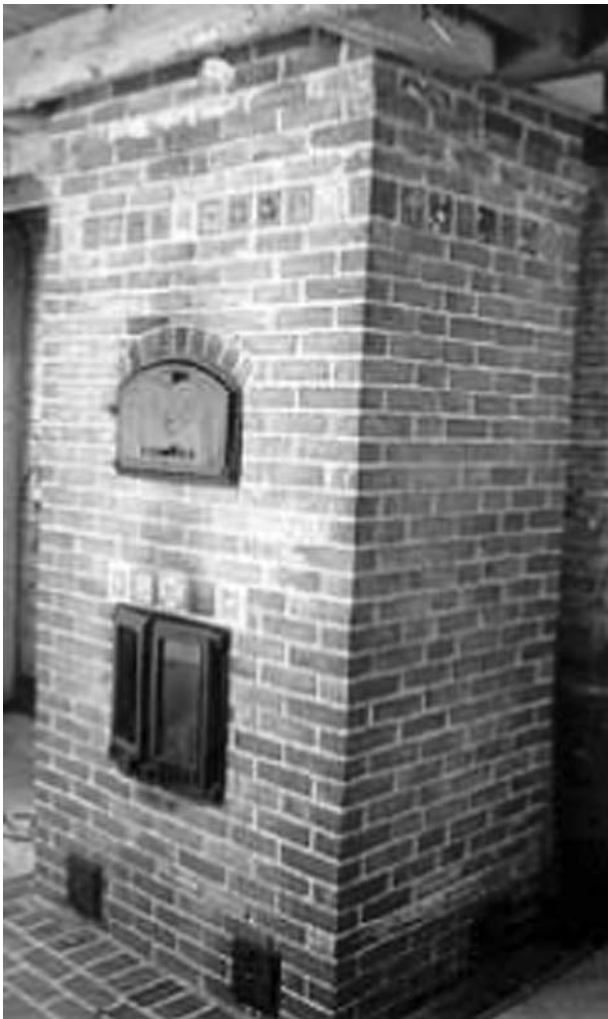
Fig. 4 Finnish stove (Courtesy of Peter Moore Masonry, Inc.). Source: From http://www.vtbrickoven.com/masonry/masonry.html
