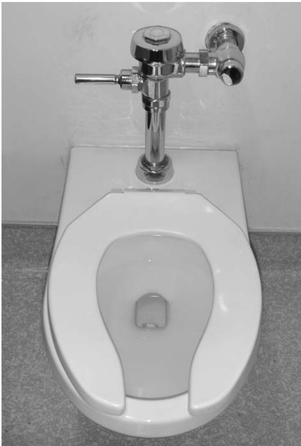
Fig. 4 Flush valve toilet.
