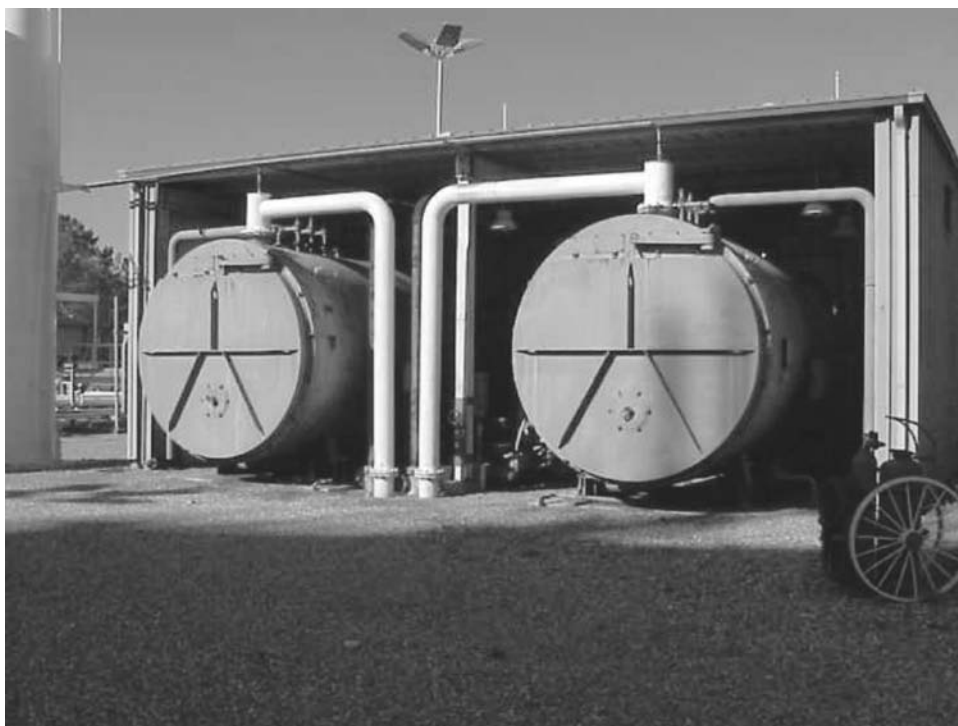
Fig. 4 Remote boilers used in regasification process.
