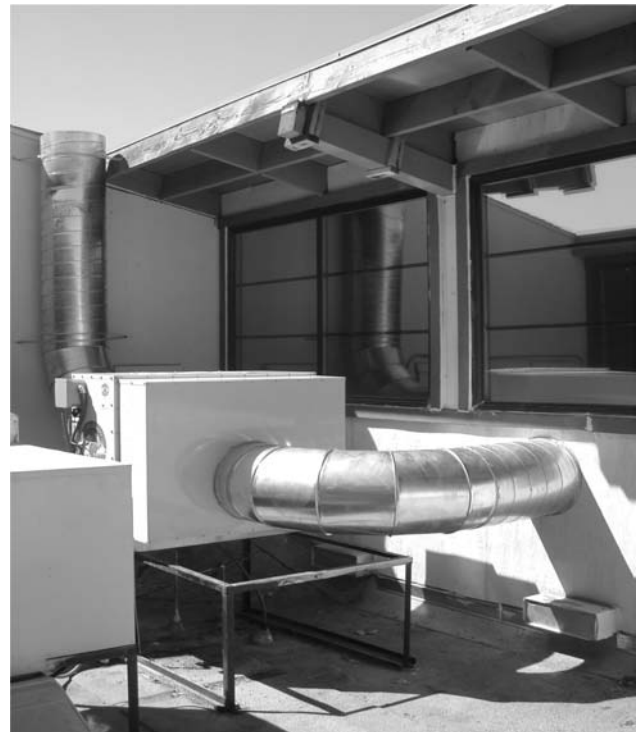
Fig. 18 Coolerado Cooler installation at a school in Sacramento, California. Source: From Sacramento Municipal Utility District (see Ref. 7).
