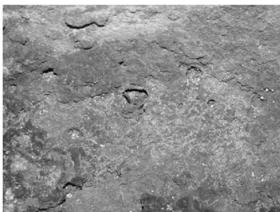
FIGURE 2.3 Close view of the inside thick scale showing areas of localized rupture leading to hole formation.
