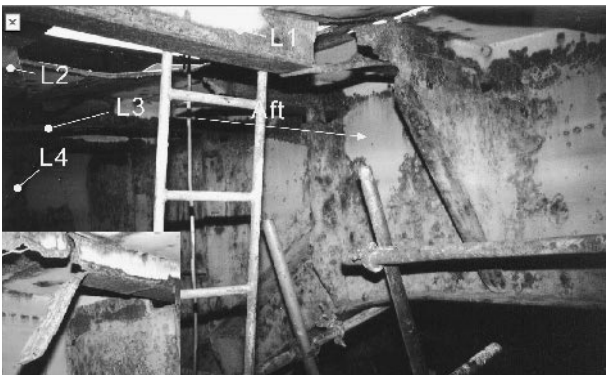
FIGURE 25.4 Heavily corroded under-deck area of M. V. Castor [2].
