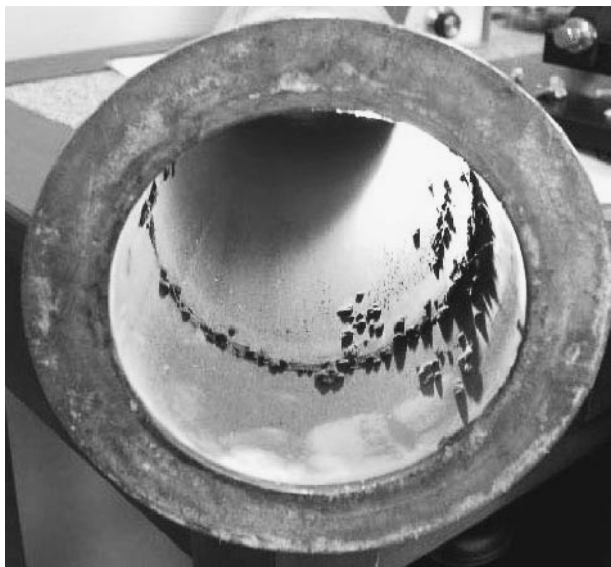
FIGURE 27.14 Tuberculation corrosion inside of a stainless steel pipeline used to transfer 180 °F hot water for heating mixing vessels.
