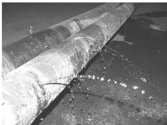
FIGURE 2.1 The leaking pipes of the NG Feed Pre-heater Coil. Water-leaks during testing are seen.
