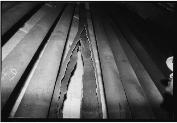
FIGURE 2.9 A close-up of the top portion of the reformer tube crack extending into the second segment from the bottom across a butt weld.
