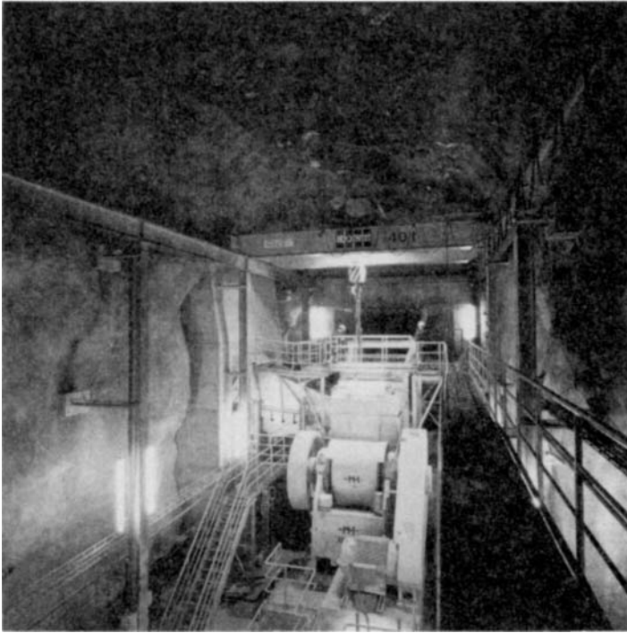
FIGURE 12.4. Underground installed crushers. By courtesy of Wolfram Bergbau und Hüttenges. m.b.H., Austria.
