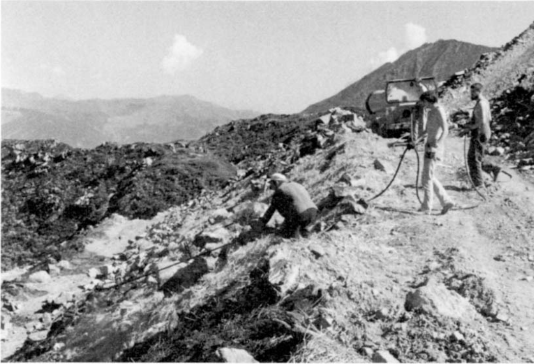
FIGURE 12.3. Reclamation of the open pit mine area. By courtesy of Wolfram Bergbau und Hüttenges. m.b.H., Austria.
