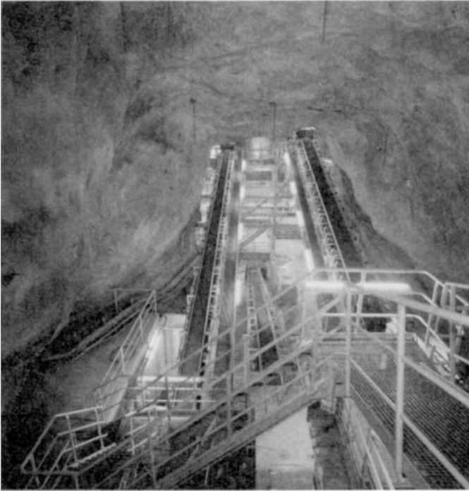
FIGURE 12.5. Underground conveyer belt connection to the ore dressing plant. By courtesy of Wolfram Bergbau und Hüttenges. m.b.H., Austria.
