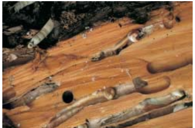
Shipworms ( Bankia setacea ) in fallen piling. Without being detected, shipworms can drill through lumber until it resembles a honeycomb and is rendered unfit for use. (Photo by Gary Gibson/Photo Researchers, Inc. Reproduced by permission.)
