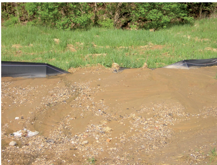
Fig. 11.1 Sediment accumulation above silt fences can overtop them under concentrated flow erosion (Courtesy C.J. Gantzer, Univ. of Missouri, Columbia, MO)
