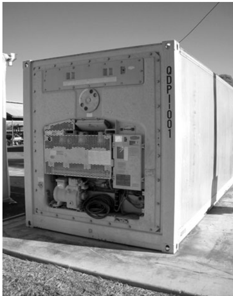
Fig. 7.1. A refrigerated shipping container capable of use for in-transit quarantine disinfestation treatment at a temperature precision of \pm 0.5^{\circ}\text{C} . The power source is mains power from the ship's supply or a land source. A data recorder (upper right of refrigeration unit) provides a charted history of temperatures over the transit time at a number of locations within the container.
