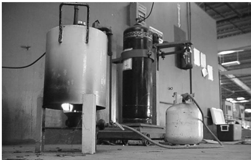
Fig. 10.3. Gas delivery equipment needed for a commercial fumigation with methyl bromide (black tank). The large tank is for heating the methyl bromide to ensure its gaseous form before entering the fumigation chamber (note flame at bottom). The small tank is the propane fuel source.
