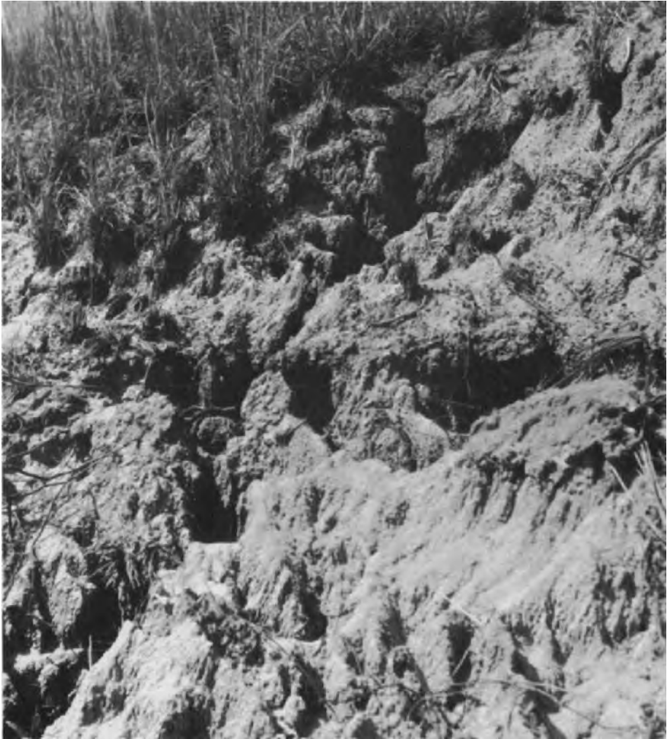
Fig. 86. Slope erosion caused by heavy rain on a road excavation site on permeable material (Ghana). (Photo J. Jeník.)
