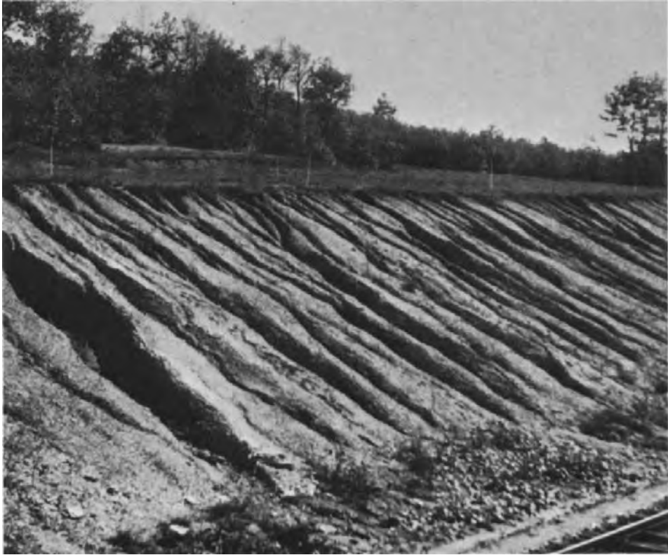
Fig. 89. Railway excavation slope consisting of loamy to sandy gravel material destroyed by rill erosion (Bulgaria). (Photo D. Zachar.)
