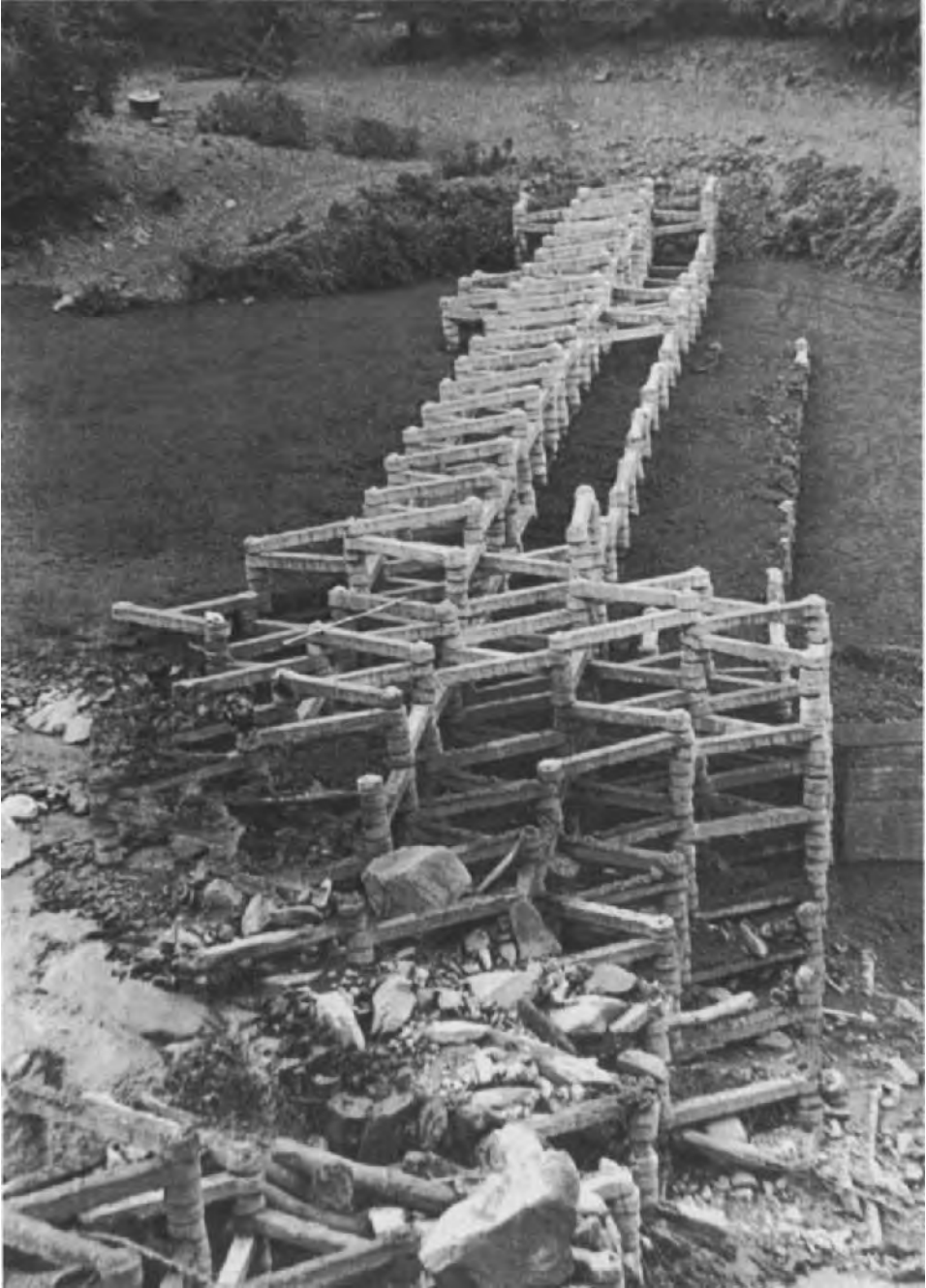
Fig. 159. Retention barrier (height 9 m, length 100 m) as a protection against mud flows in Georgian SSR. (Photo S. G. Totashvili.)
