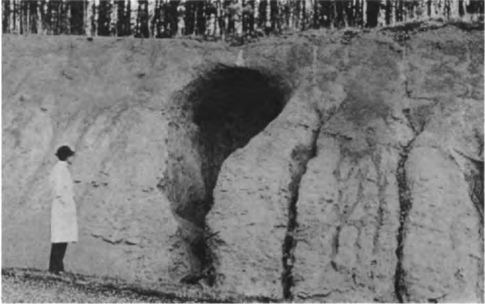
Fig. 34. Erosion funnel – the beginning of tunnel erosion on the excavation site of a road (Cataula, Oregon, USA). (The author's collection of photographs.)
