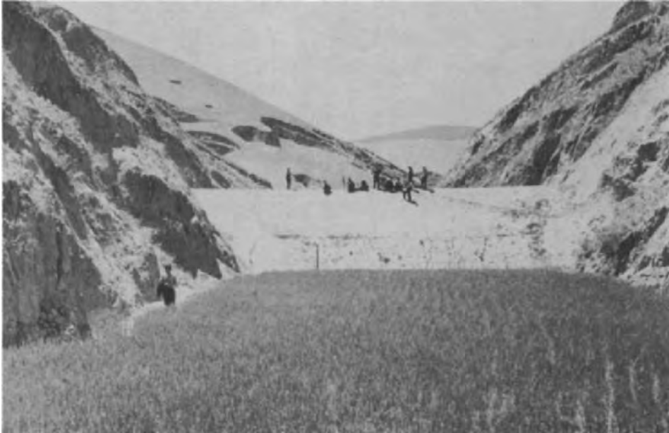
Fig. 161. The first step in the prevention of erosion is the stabilization of river courses, the control of floods and gullies. The system of earth dams shown in the picture prevents vertical erosion, and therefore also inhibits the erosion of adjacent slopes. (The author's collection of photographs.)
