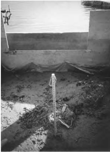
The back of a dump truck filtration system looks something like this: a weir (made of \frac{3}{4} inch plywood) for the overflow and filter fabric to prevent sediment loss from under the weir. Water drains from the bottom as well as over the weir.
