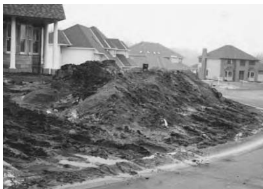
Erosion control at construction sites is critical to reduce sediment and nutrient transport to streams, wetlands, or lakes.
