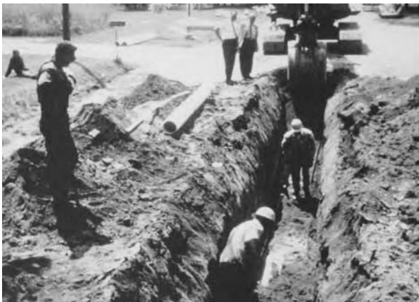
Conventional centralized wastewater treatment consists of gravity sewers and centralized wastewater treatment alternatives. Here, gravity sewers are being installed. (From USEPA, 1980a.)
