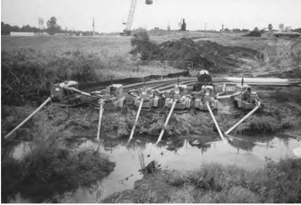
Pumping down the lake in order to work on the lakebed is an option if there is no outlet control structure.
