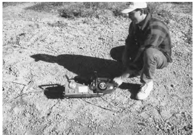
To pull the slusher out of the lake, you can use a winch device. This winch is powered from a chainsaw engine and can pull more than 2000 pounds. The winch is anchored with a land anchor. The land anchor is screwed into the ground.
