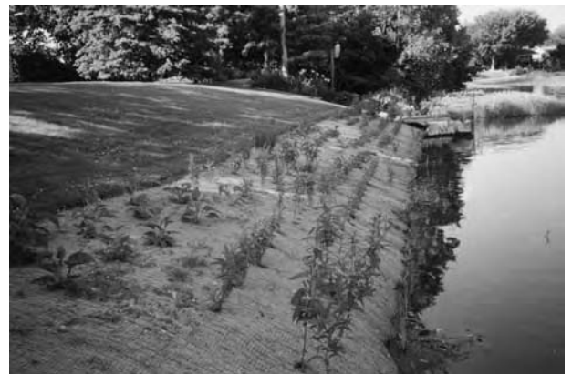
The erosion control solution was a biostabilization approach. The lakeshore was regraded, an erosion control mat was laid down, and vegetation was planted into the mat. (From Bonestroo, Rosene, Anderlik & Associates, St. Paul, MN., 2000.)
