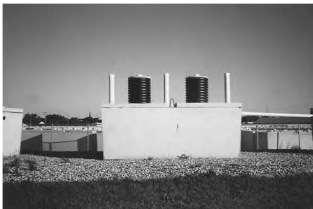
The septic tank. This is what goes in the ground.
