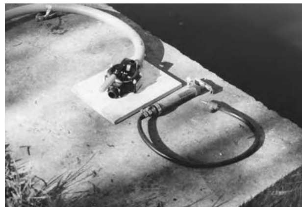
Hand pumps pump the alum slurry through the manifold.
