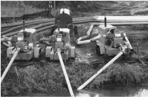
Another way to draw down a lake is to pump it down. Using several pumps will speed the job. Costs can go as high as $1000 per day, depending on the amount of water pumped and where it is being discharged.
