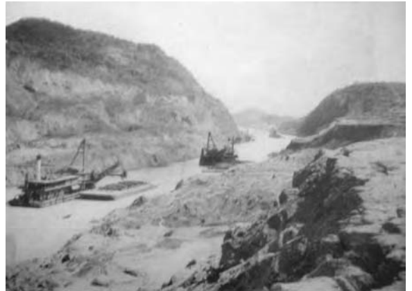
A fleet of 15-cubic-yard dipper dredges working on the Gailard Cut, Panama Canal, in 1915. (From Excavating Engineer , Vol. 12, 1916.)
