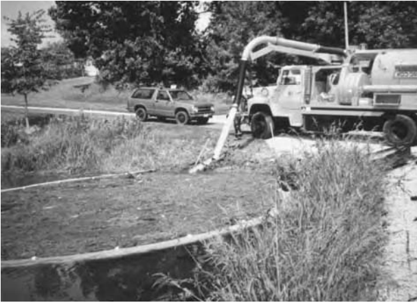
The City of Eagan (Minnesota) uses a sewer vacuum truck to suck up the collected filamentous algae. It would also work for duckweed.
