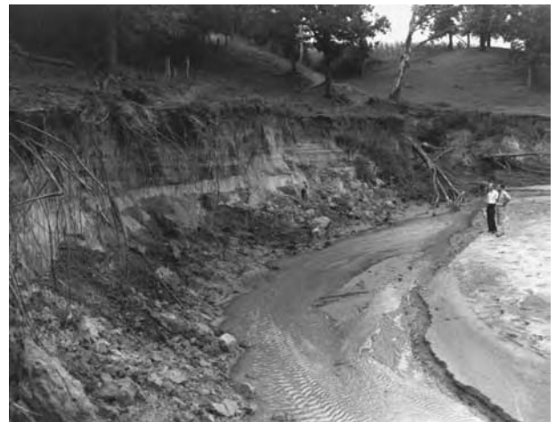
Even streams with low base flow can cause significant bank erosion. (From USDA)
