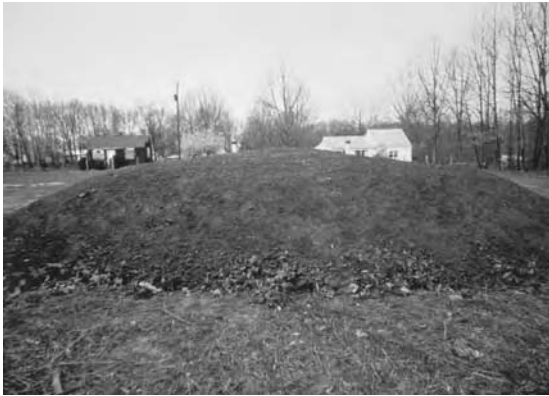
Mound systems eventually become part of the landscape. However, they are susceptible to leaking at the toe. (From USEPA, 1980a.)
