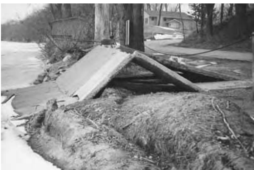
To accommodate the force of the ice push, flexibility is the key. This boat launch was folded up like an accordion. Even boat launches can be designed to be flexible using reinforced concrete strips connected by chains that can be repositioned in the spring. For other lakeshores, biostabilization-based projects are more easily repaired than inflexible revetments.
