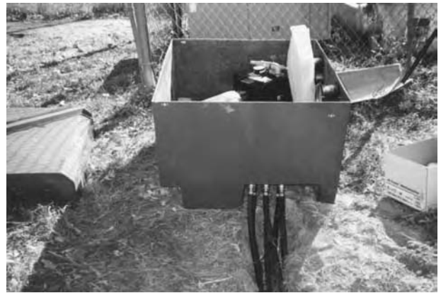
Like the conventional aeration systems described in Chapter 2, the air compressors used for winter aeration are contained in onshore housing, with air lines going out into the lake to diffuser heads.
