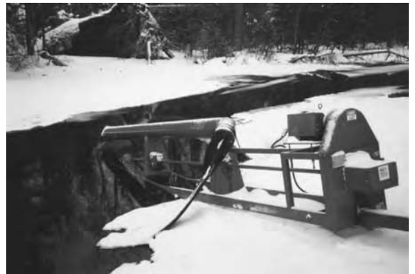
The pump-and-baffle system can be temporary or permanent. This is a temporary installation. The intake is placed in shallow water and water is pumped up to a baffle component. In this case, the objective was to boost oxygen levels in a stream that was leaving a lake low in oxygen. Then the re-aerated stream water flowed into the downstream lake and gave it an oxygen boost. (From Frank Splitt, Ballard Lake, WI.)
