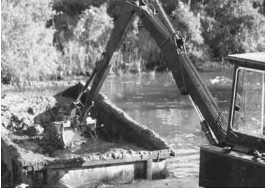
A muck barge is needed to haul sediment back to land when working away from shore.
