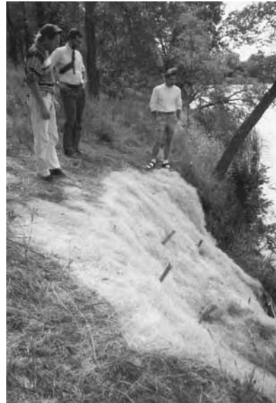
This lake bluff erosion problem was addressed with a temporary brush shoreline wavebreak and erosion control matting. However, the brush wavebreak was not protecting the toe and, without reshaping the bank, the bluff probably will not stabilize.
