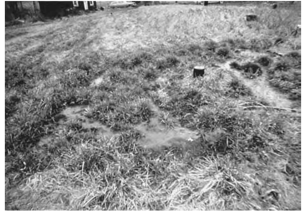
A soggy drainfield with standing water is a sign of a surface failure. This problem needs to be fixed immediately. (From USEPA.)
