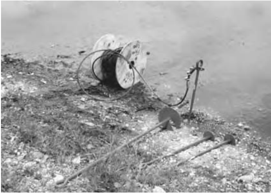
The basic components of a cable and pivot are a land anchor (used as a pivot) and a length of cable about 100 feet long with a \frac{5}{16} -inch diameter.
