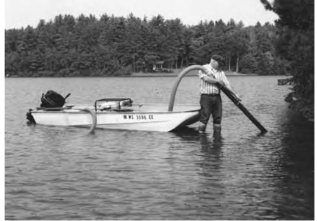
A centrifugal pump (3-inch intake) generates a discharge to remove silt and muck buildup. It can be placed in a boat and can easily be moved around.
