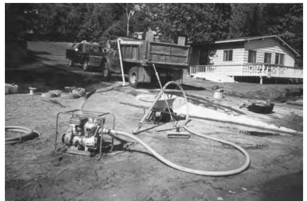
You can use the box of a dump truck as a movable holding/dewatering area. Truck boxes will hold 6 to 8 cubic yards of material.
