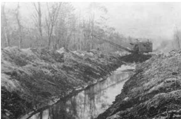
Digging drainage ditches was common in the early 1900s to drain wetlands to create more farmable acres. The purpose of this 3-mile ditch was to drain a wetland to reduce bog-stained water from entering the water supply of Bridgeport, Connecticut. (From Excavating Engineer , Vol. 13, 1917.)
