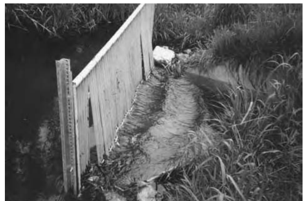
Although this barrier is permanently installed, the gates swing in 6-inch sections to allow debris to pass through. This keeps most of the carp from swimming back into the lake.
