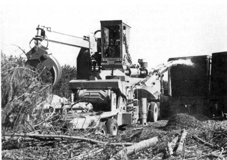
Figure 19.11 An in-woods chipper can fully utilize the woody biomass on the site and reduce subsequent reforestation costs.
