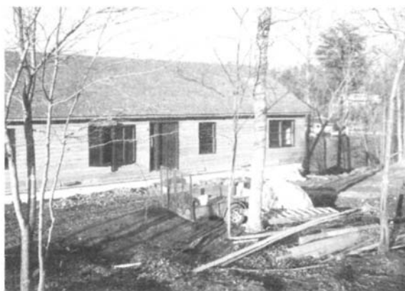
Figure 22.8 Construction activity can have severe negative impacts on root-zones of trees.
