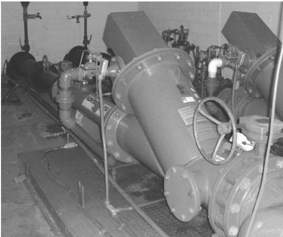
Fig. 7.10. Water pumps are usually placed in specially constructed buildings that protect them from weather damage.
