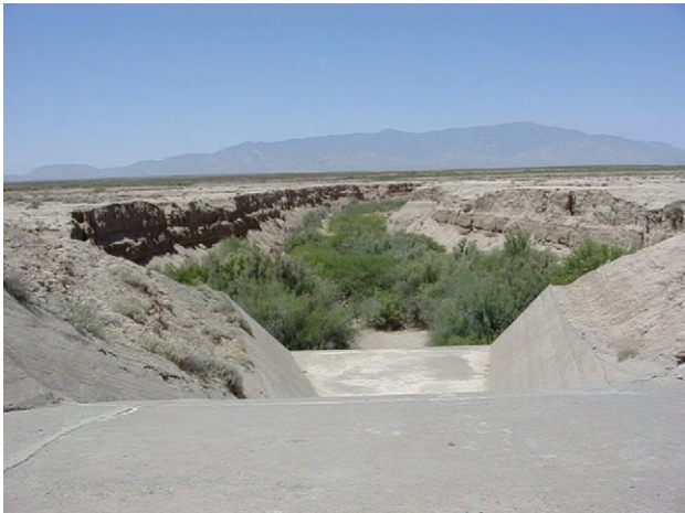
FIGURE 15.14 Erosion control structure at the head cut of a large gully. This structure has stopped growth of the gully by providing a stable channel to drop the water into the bottom of the gully.
