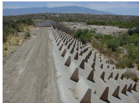
FIGURE 15.13 Erosion control structure at the foot or bottom of a large gully. Sediment has filled in on the upstream ( left ) side of the structure, filling the gully above the structure.
