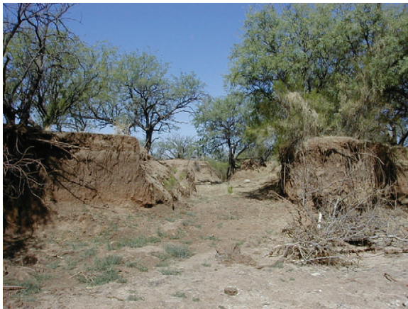
FIGURE 15.9 Gully erosion. (Photo by Walworth.)
