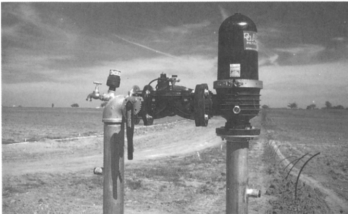
Figure 7.9 In this system, a manual clean disc filter is installed with the valve at the entrance to each irrigation block as a back-up to the main filters (system under construction)
