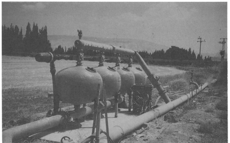
Figure 7.8 Media filtration unit. Multiple tanks are necessary to accommodate the required flow rate, and to provide for automatic backflushing.
