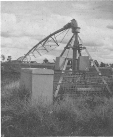
Figure 6.9 Pivot end of a centre-pivot irrigator. Electricity and water are delivered to the pivot point, then along the machine. This older style machine has medium pressure sprinklers mounted on the sprayline.
