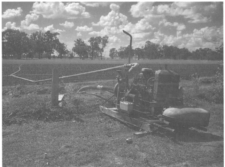
Figure 8.4 This is a portable (skid-mounted) diesel powered centrifugal pump delivering water from a channel to a hand shift spray system. Although it looks a bit untidy, it is fitted with electric start and shut-down protection. It should be placed on a firm level pad
