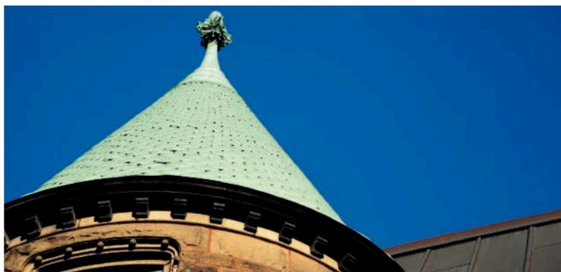
This copper roof has turned green because the metal has reacted with gases in the air (including carbon dioxide gas in this case) and has become tarnished
