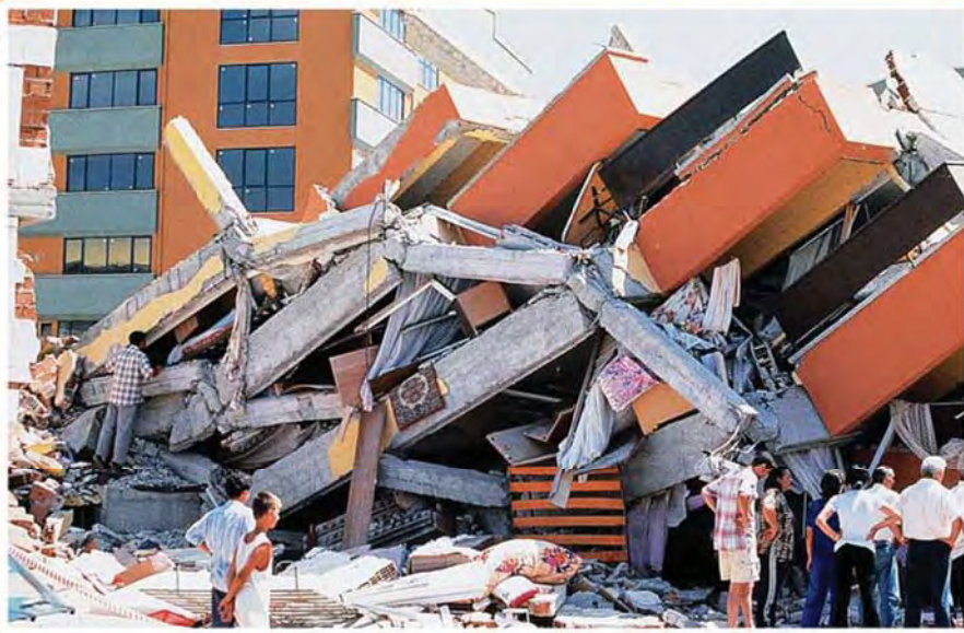
The quake destroyed 85,000 buildings. Many of the buildings were poorly constructed with inferior building materials. Floors of buildings “pancaked” and crushed the residents.
