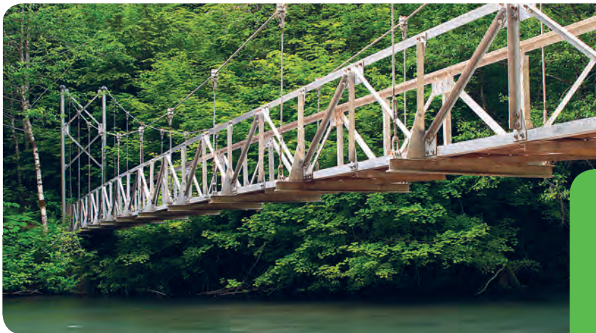
Ohanapechosh River A suspension bridge on the Grove of the Patriarchs Trail
