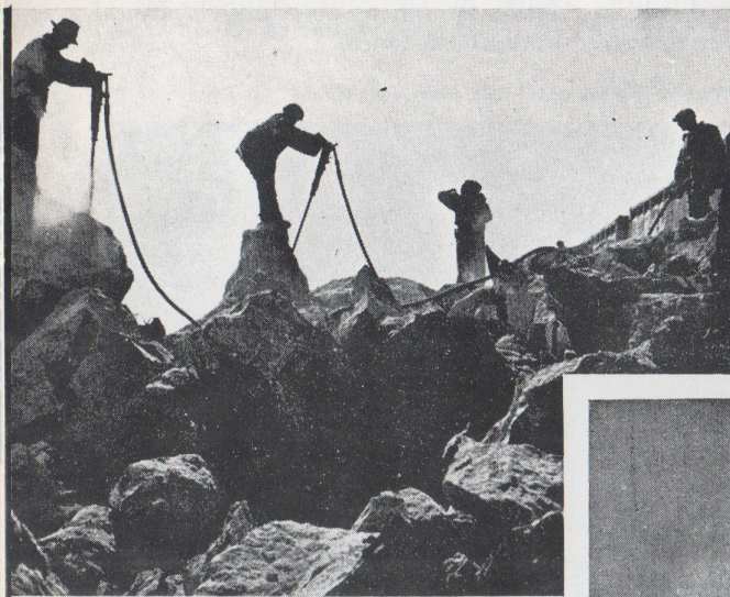
Drillers prepare to blast nitrate from the ground. The explosion makes a dramatic backdrop in the stark region
